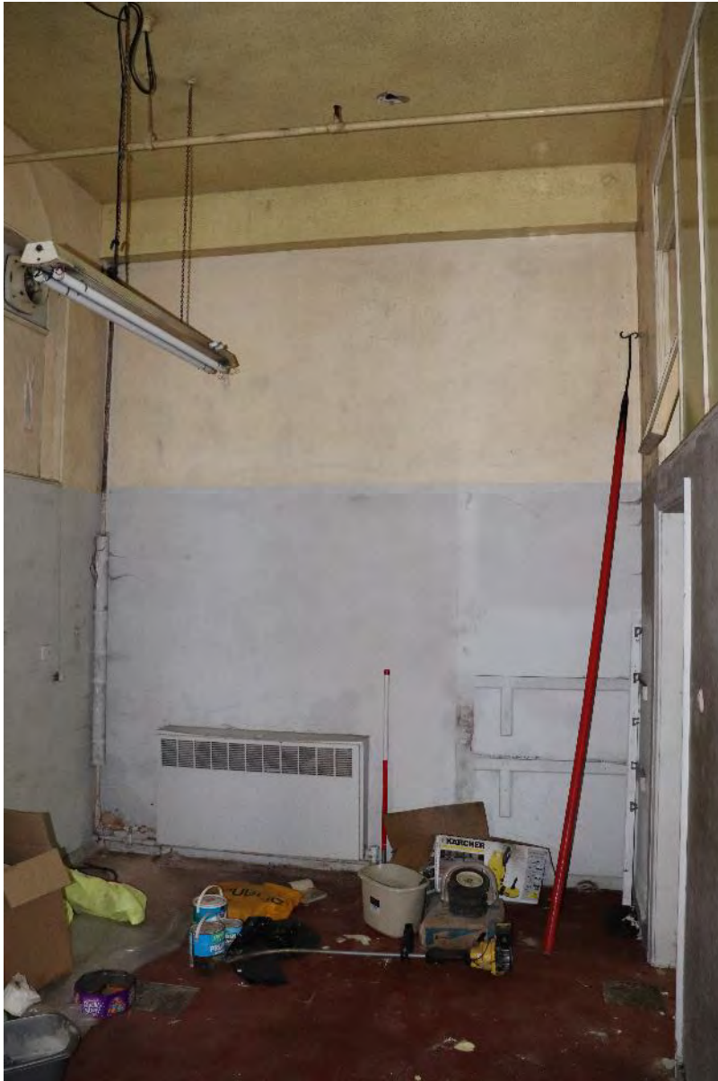
Plate 21 Phase 1 a Chenille and Yarn store ground floor, looking north-east, scale 1m
