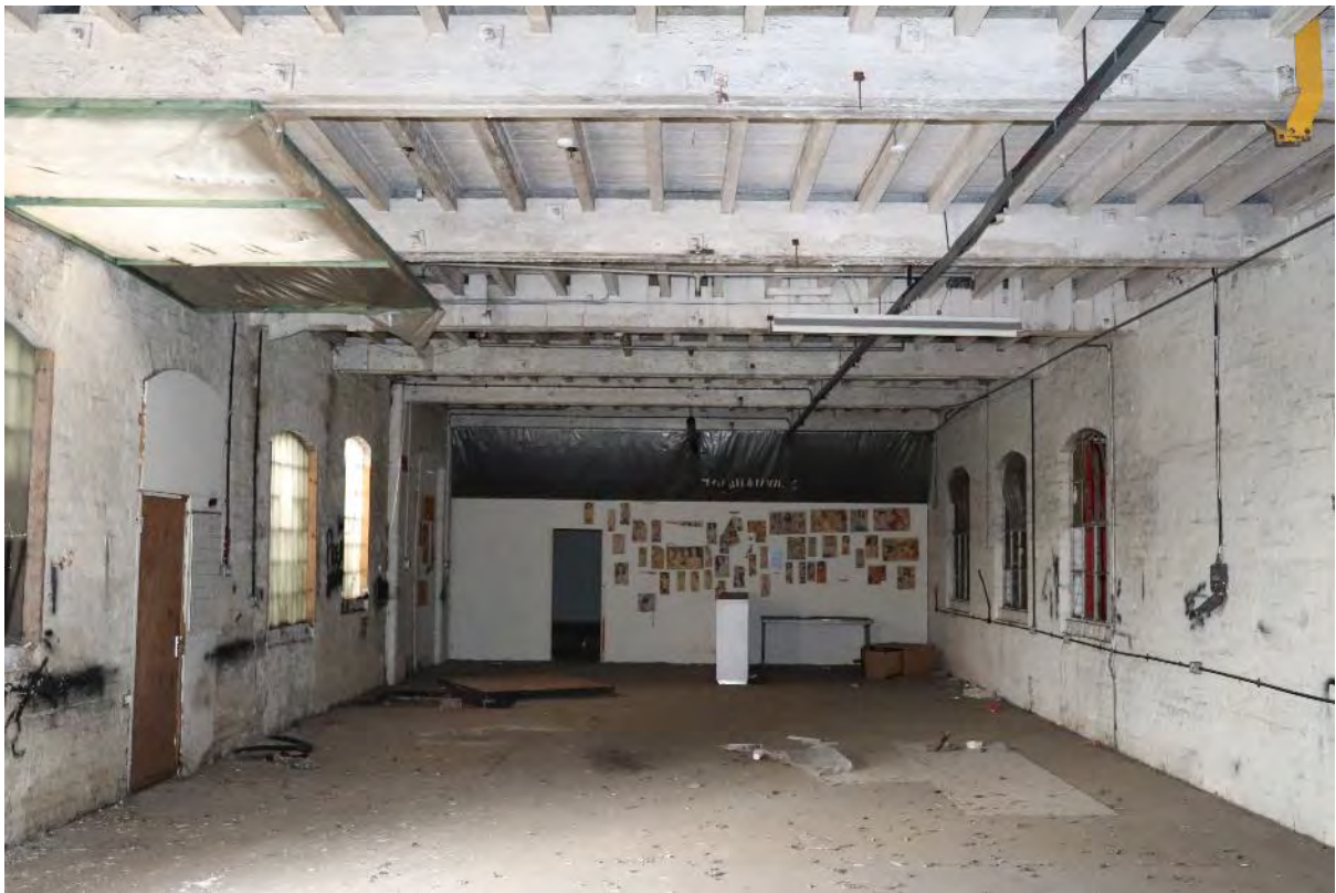
Plate 29 Duke Street north range Phase 1 b ground floor, looking south-west, scale 1m
