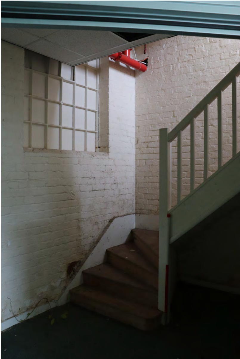
Plate 43 Phase 2 Duke Street south range ground floor later added staircase, 1m scale, looking south
