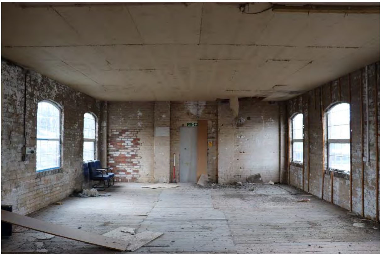
Plate 12 Phase 1a Duke Street north former gable end at first floor level from within the Phase 1b addition, looking south-east, 1m scale
