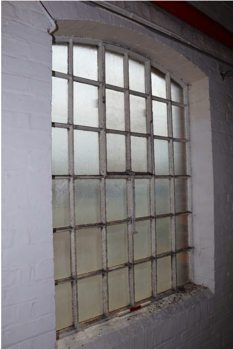
Plate 42 Phase 2 Duke Street south range first floor window, 0.3m scale, looking south-east
