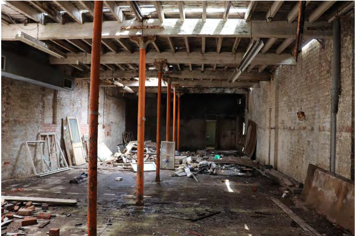
Plate 33 Duke Street north range Phase 1 b further extension, looking north-east, 1m scale
