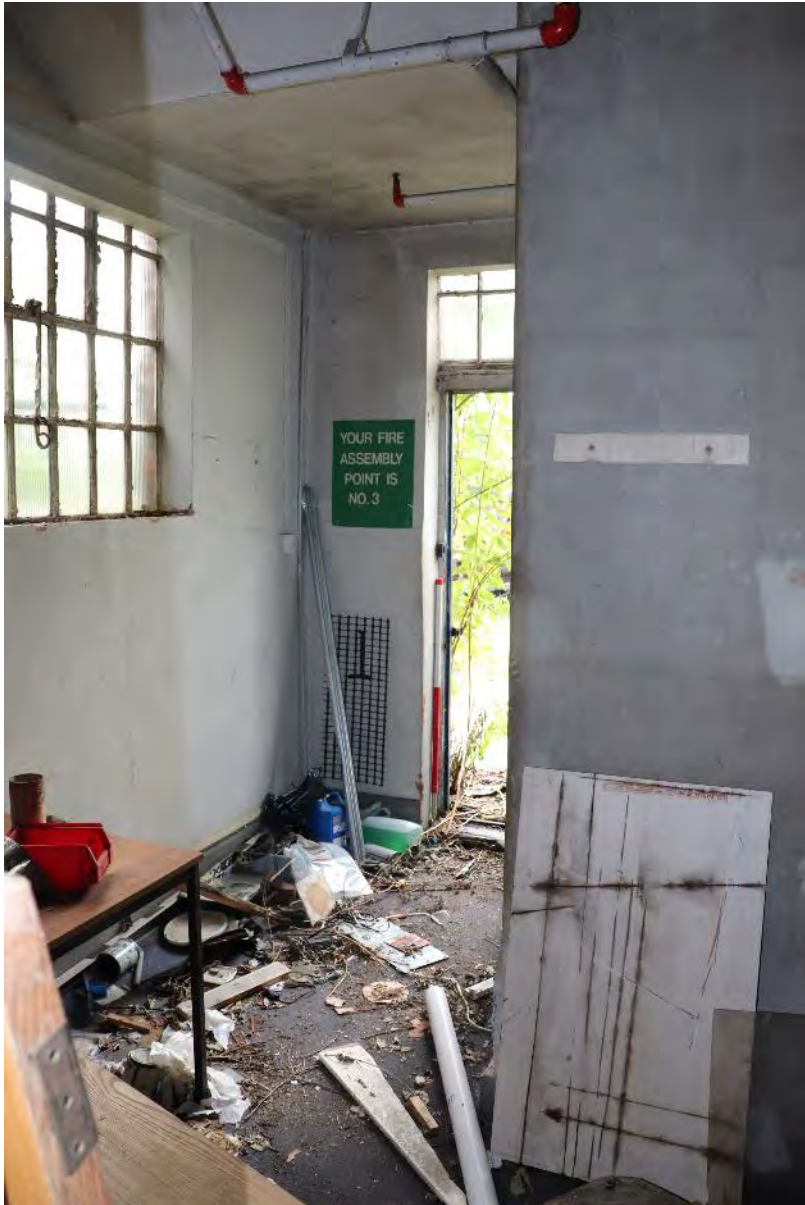
Plate 20 Phase 1 a Chenille and Yarn store ground floor, looking south, scale 1m
