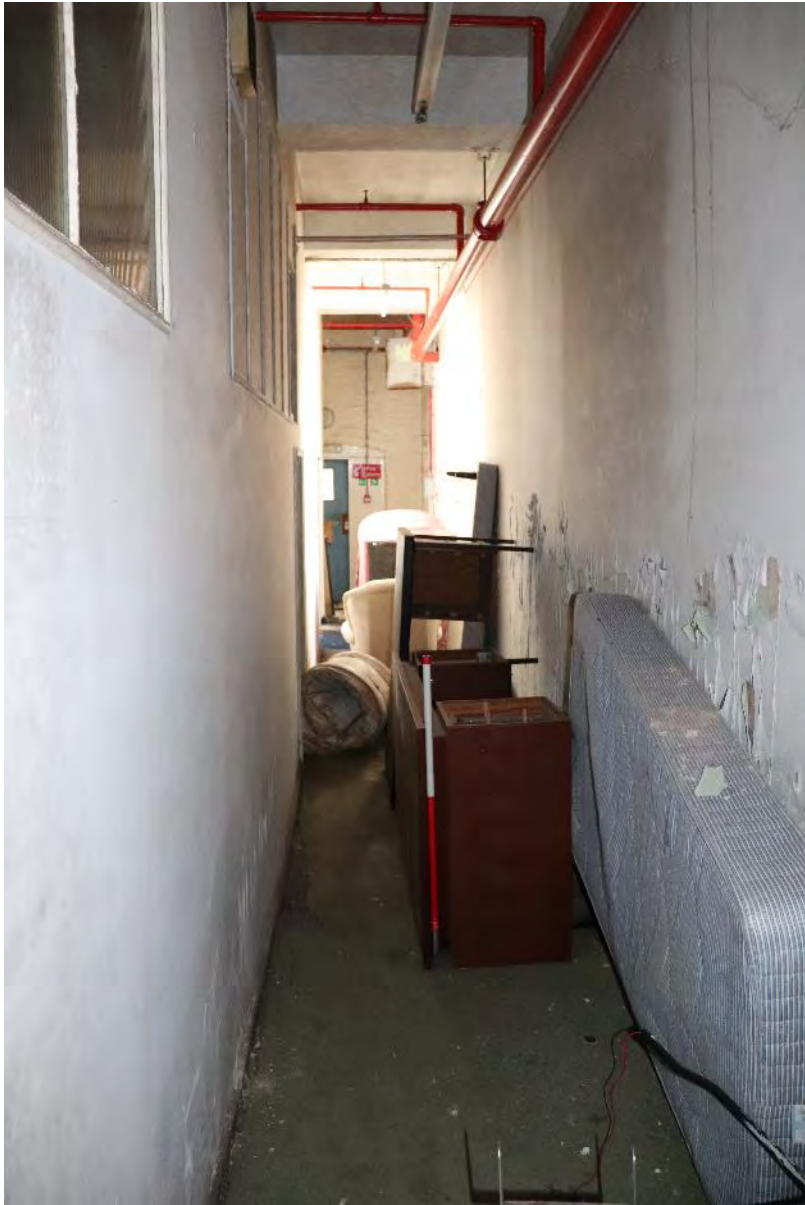
Plate 22 Phase 1 a Chenille and Yarn store ground floor, looking south-west, scale 1m
