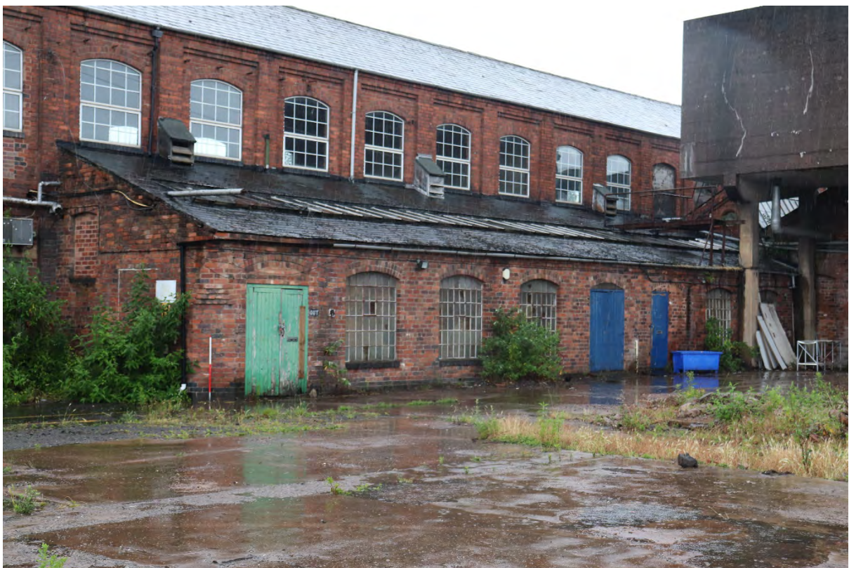
Plate 51 Phase 3 addition to the Duke Street north range, 1m scale, looking west
