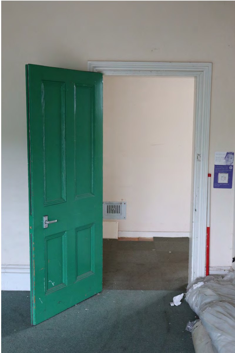
Plate 37 Phase 2 Duke Street south range ground floor original door, 1m scale, looking north-east
