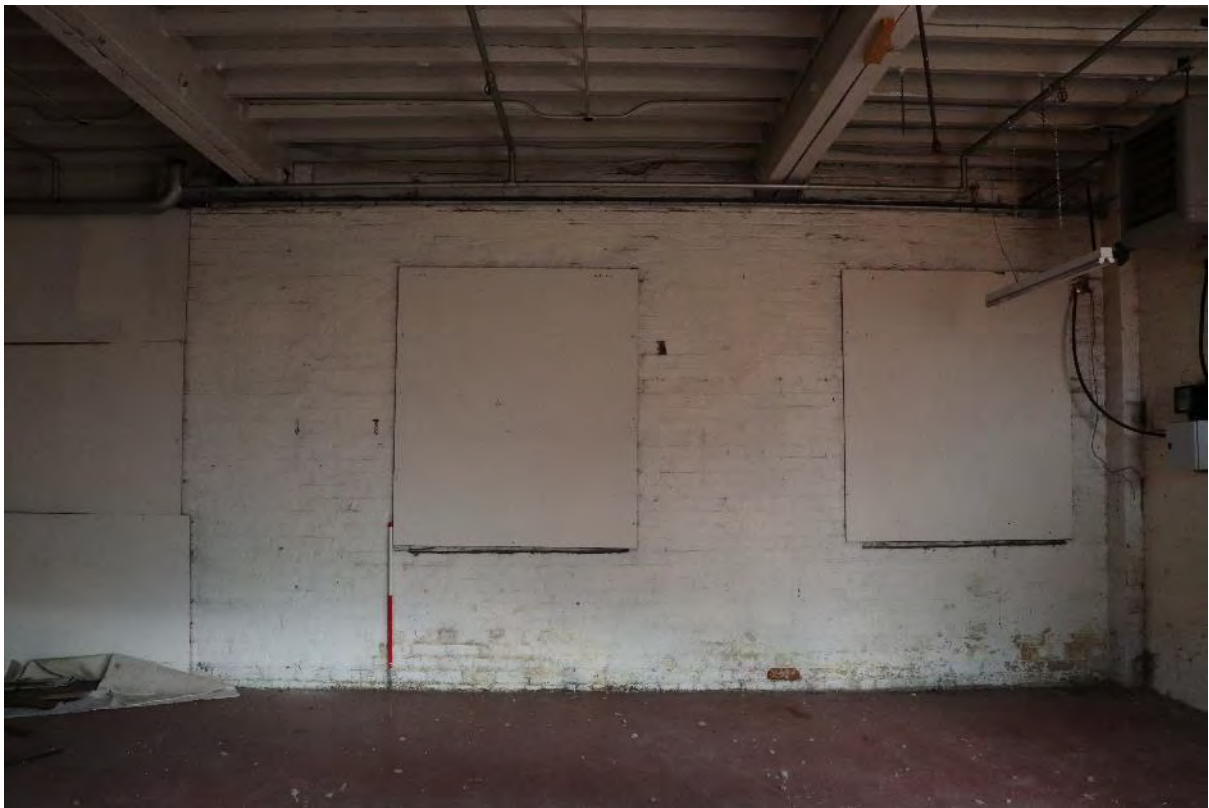
Plate 31 Duke Street north range Phase 1 b ground floor blocked former cart entrance and window, looking north-east, scale 1m
