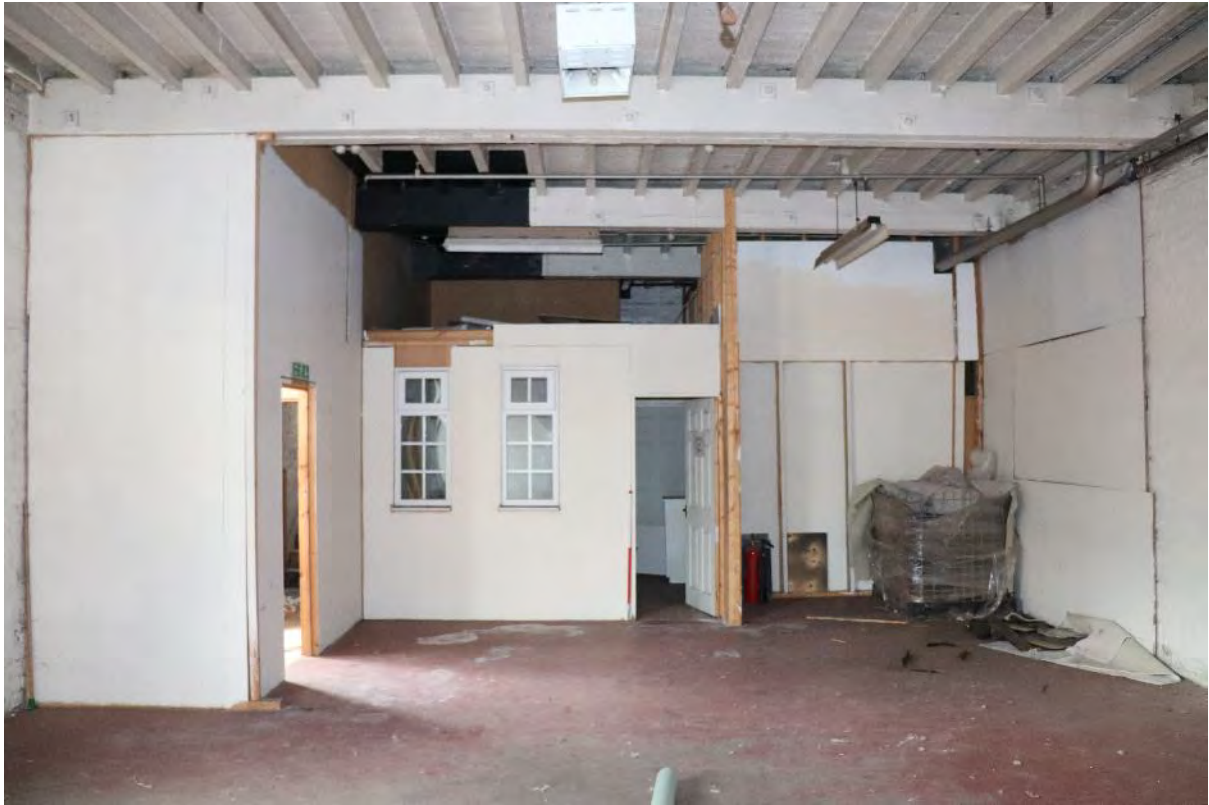
Plate 28 Duke Street north range Phase 1 b ground floor, looking north-west, scale 1m
