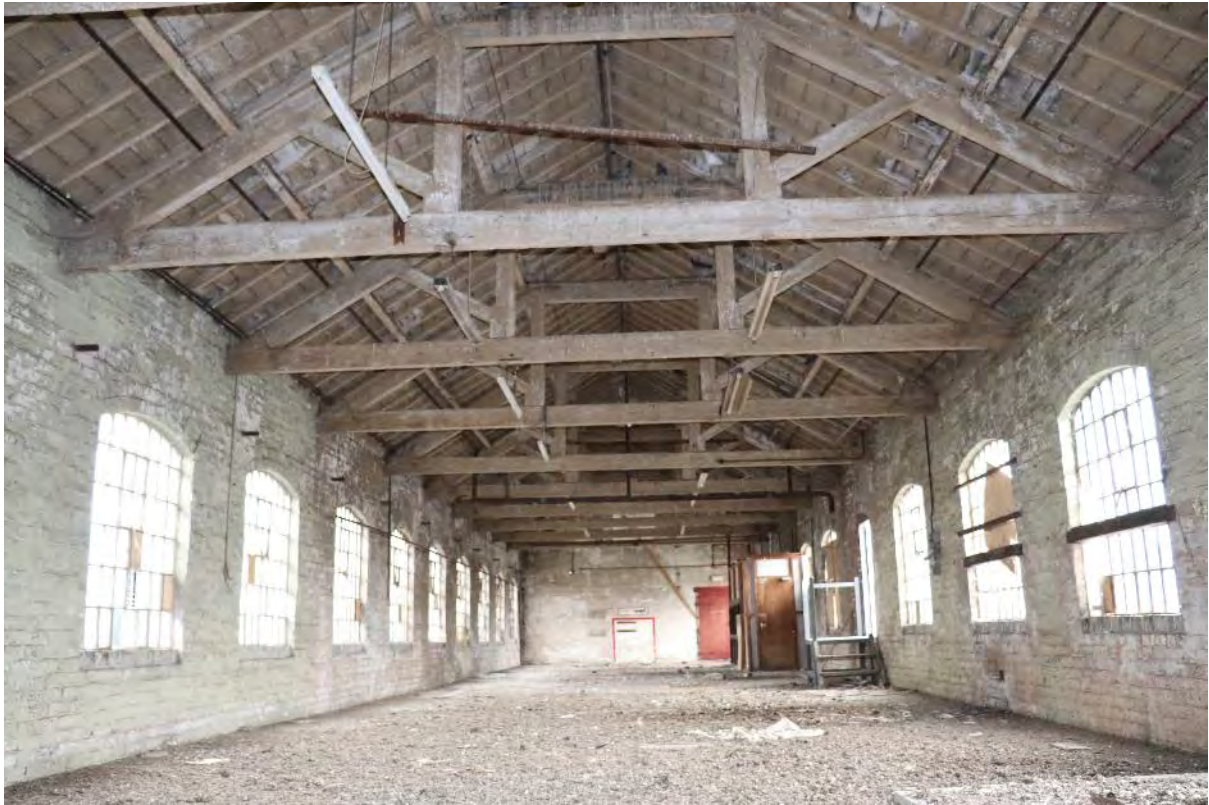
Plate 30 Duke Street north range Phase 1 b first floor, looking north-east, scale 1m
