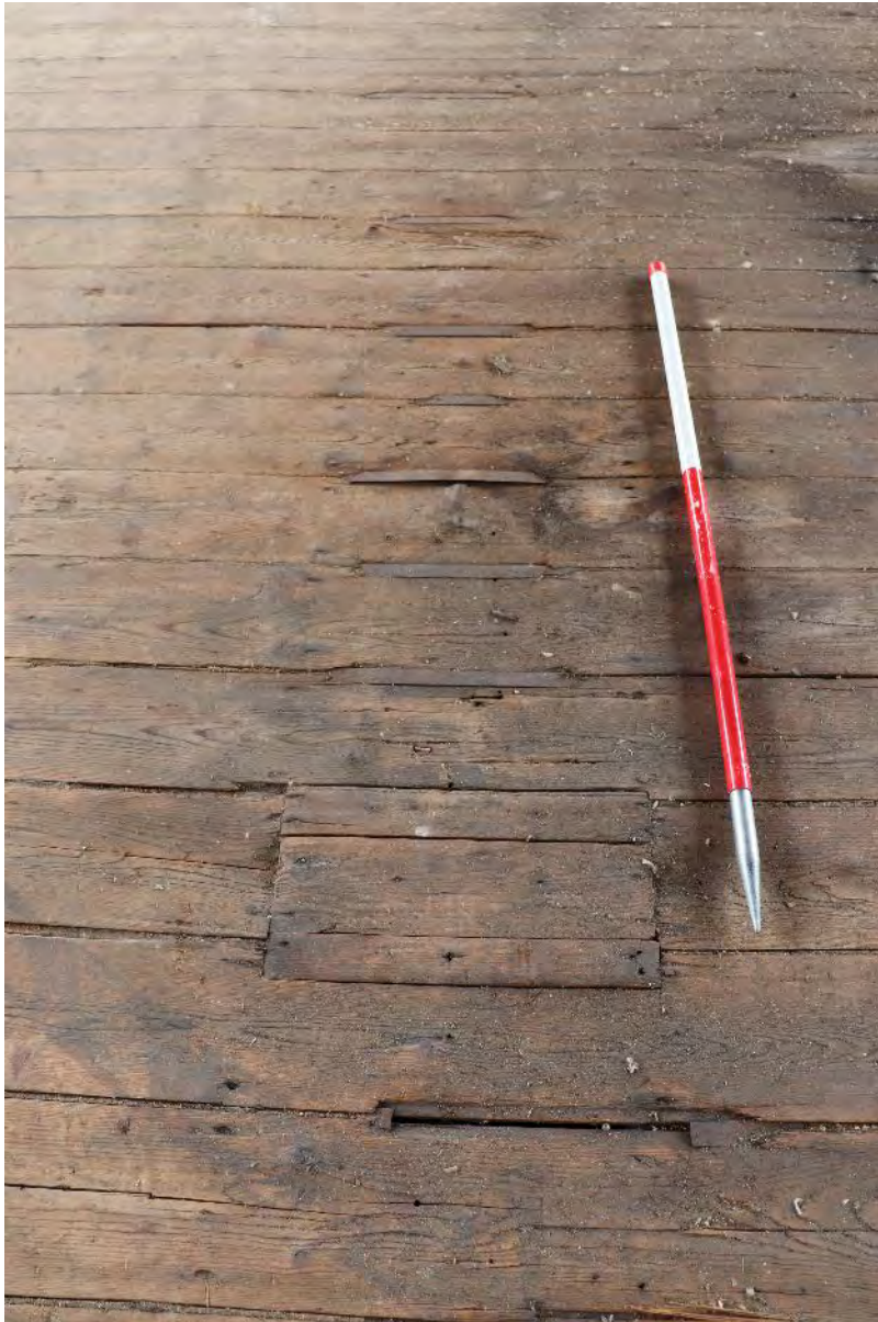
Plate 17 Phase 1a Duke Street first floor showing a wear pattern and exposed steel plates between boards, looking south-east, 1m scale
