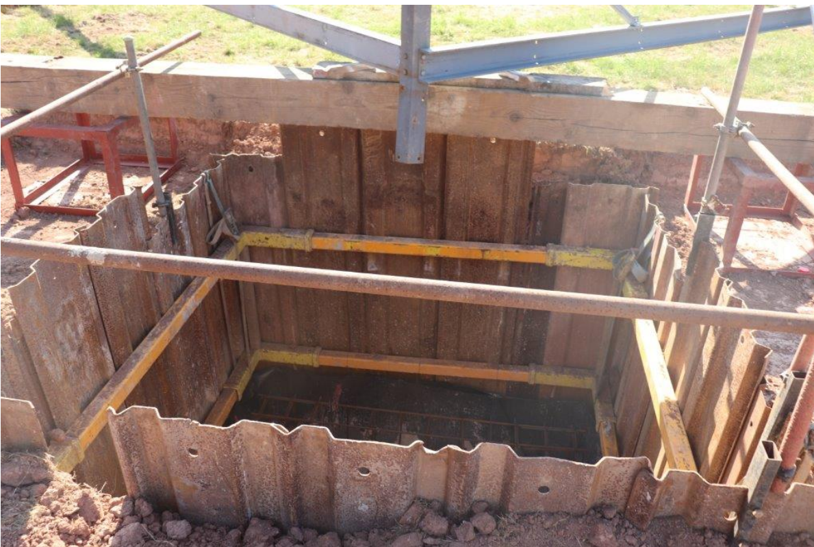
Plate 2 Example of one of pylon base pits shuttered and filled with concrete
