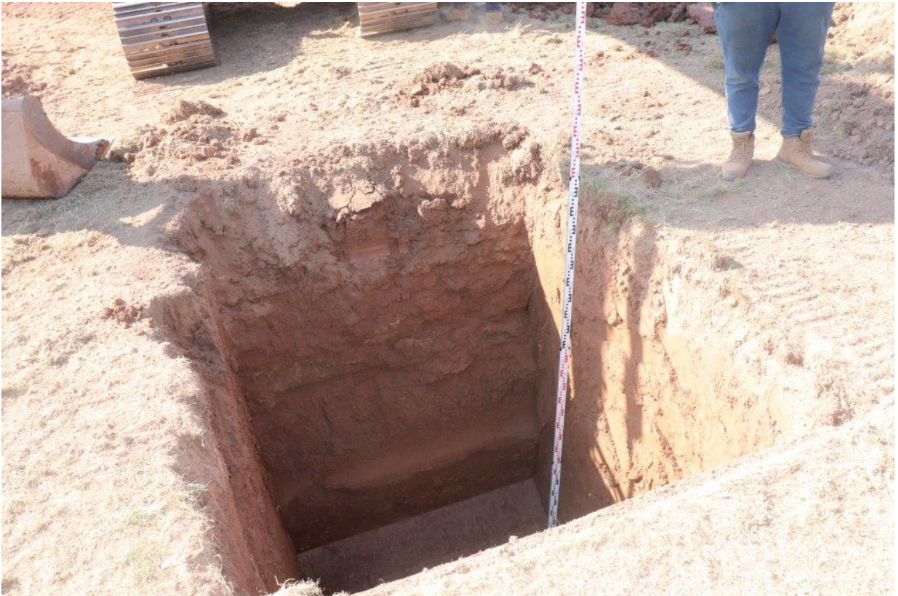
Plate 5 Test Pit 1 excavated to full depth of 3.00m showing sterile homogenous alluvial deposits above sand and gravel river terrace at base, measuring staff as scale, view south-west
