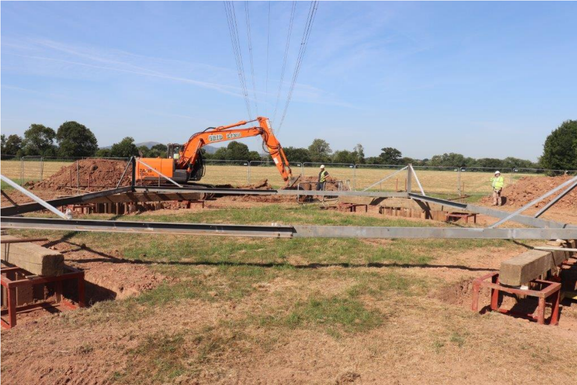
Plate 1 The pylon area showing machine in area of TP1 and existing works, view west
