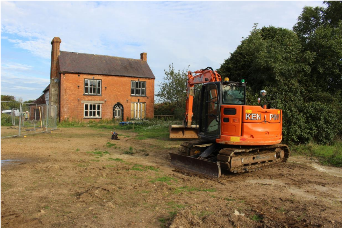
Plate 1: Site area with trenching about to commence, facing north-west towards Allesborough Farmhouse
