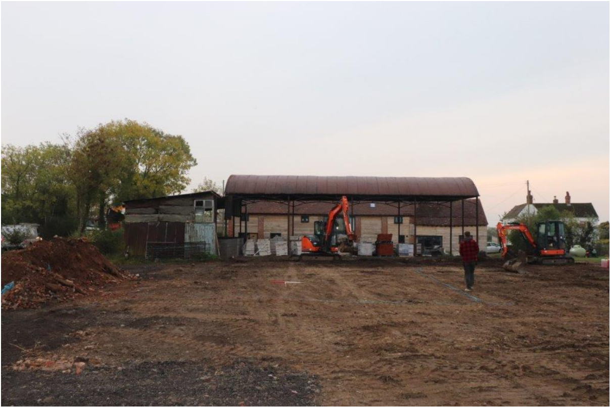
Plate 1: Site area laid out before foundation trench excavation commenced, view south-east, no scales
