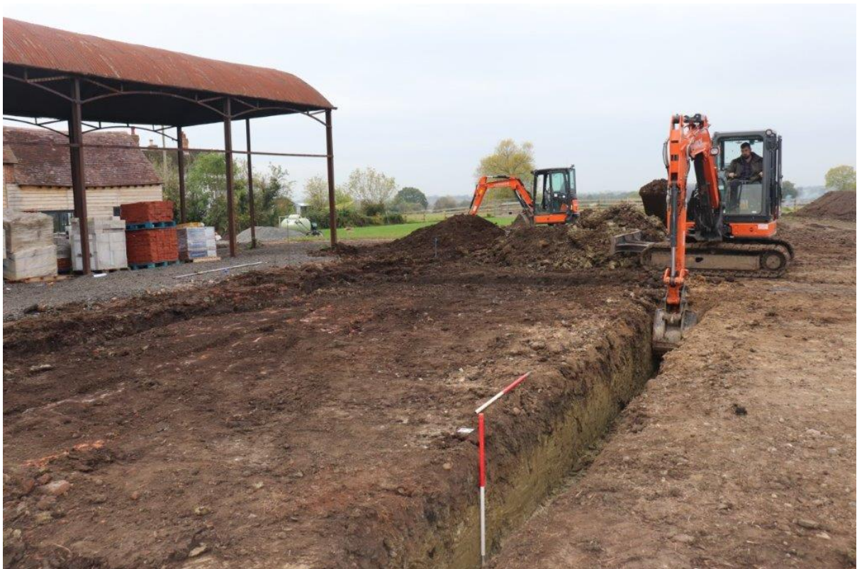
Plate 4: Central trench being excavated showing made ground and natural clays, view south, 2x 1m scales
