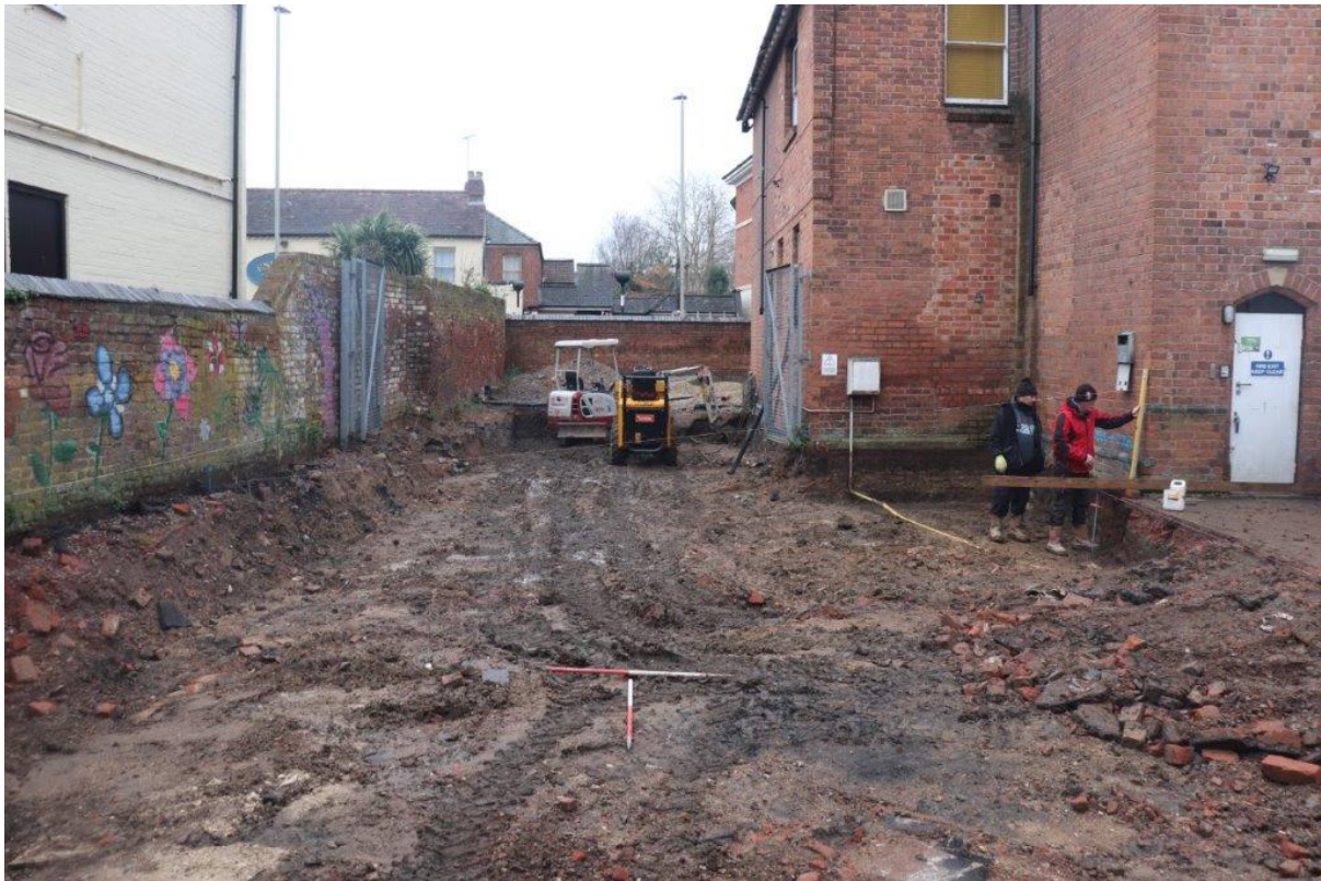
Plate 1: Setting up on site after removal of car park surface, view south; 2x 1m scales
