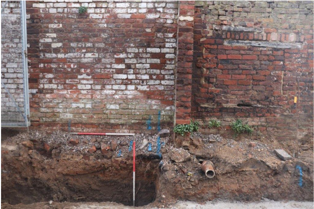
Plate 7: Southern trench after removing car park surfacing, view south; 2x 1m scales
