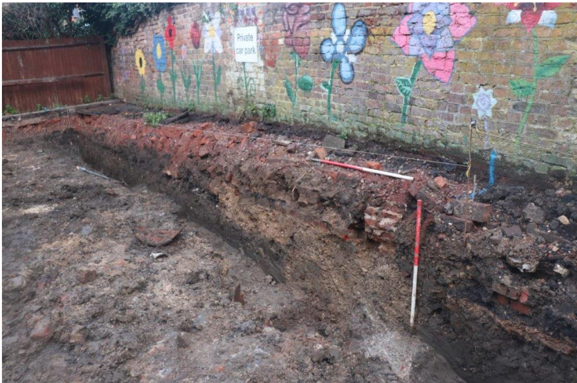
Plate 4: North-east part of site showing modern build up and walls over well 305, view north-east; 2x 1m scales
