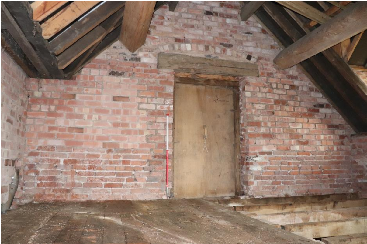
Plate 15 Phase 3a dovecote with floor level brick degradation , looking north-west, scale 1m
