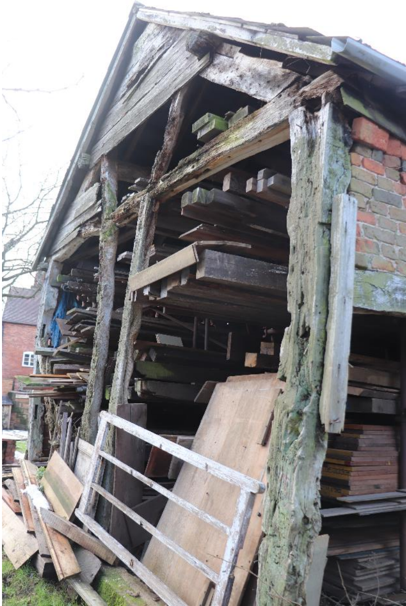
Plate 8 Phase 1 barn with empty mortice and stave holes under the tie beam, looking south-west
