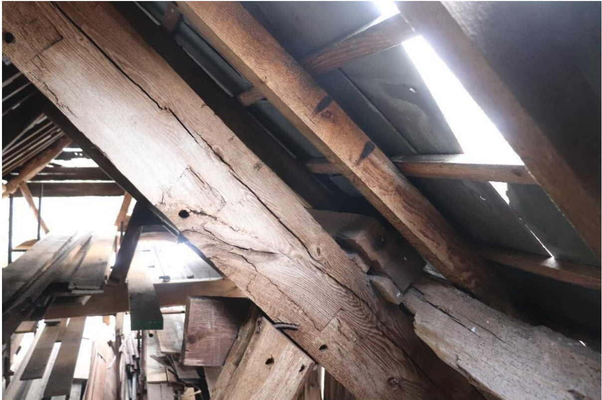
Plate 11 Phase 2 burn marks, looking east
