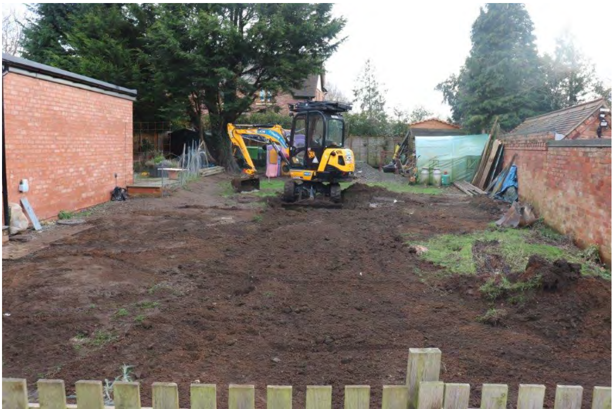
Plate 7: Trench backfilled following metal detecting of spoil and completion of works. View southeast
