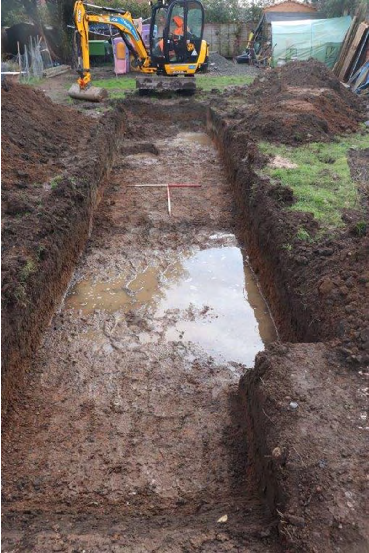
Plate 3: Trench fully excavated with groundwater and, quarry pit 104 in distance. View southeast with 1m scales
