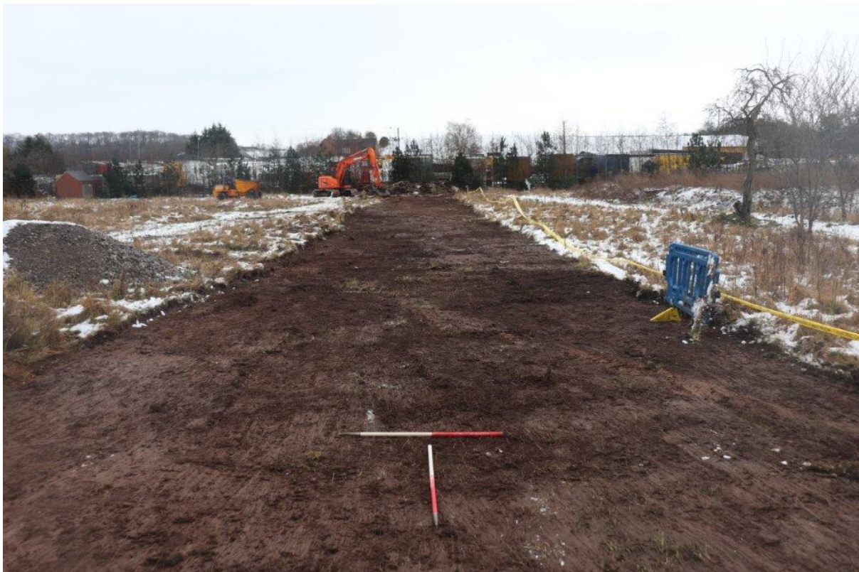
Plate 2: Site topsoil strip in southern limit of the site. 1m scales looking east
