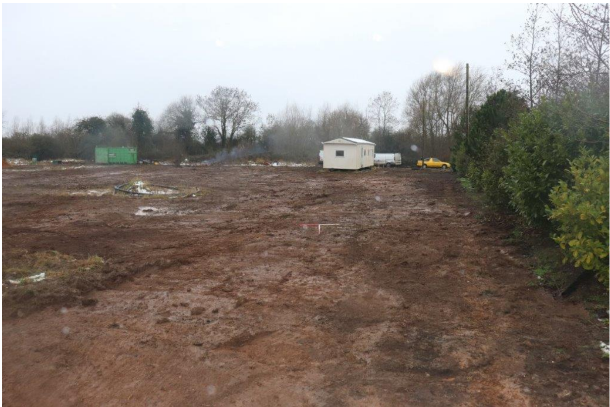
Plate 6: Topsoil stripped over northern limit the site, looking west with 1m scales
