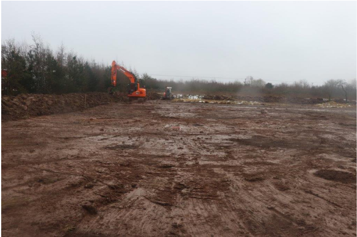
Plate 7: Topsoil stripped over the eastern side of the site, looking south with 1m scales
