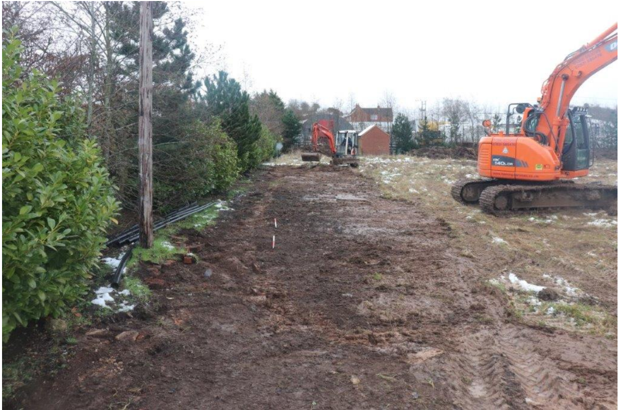
Plate 5: An electric cable service trench showing as a pale band of fill running towards the substation. 1m scales looking east.
