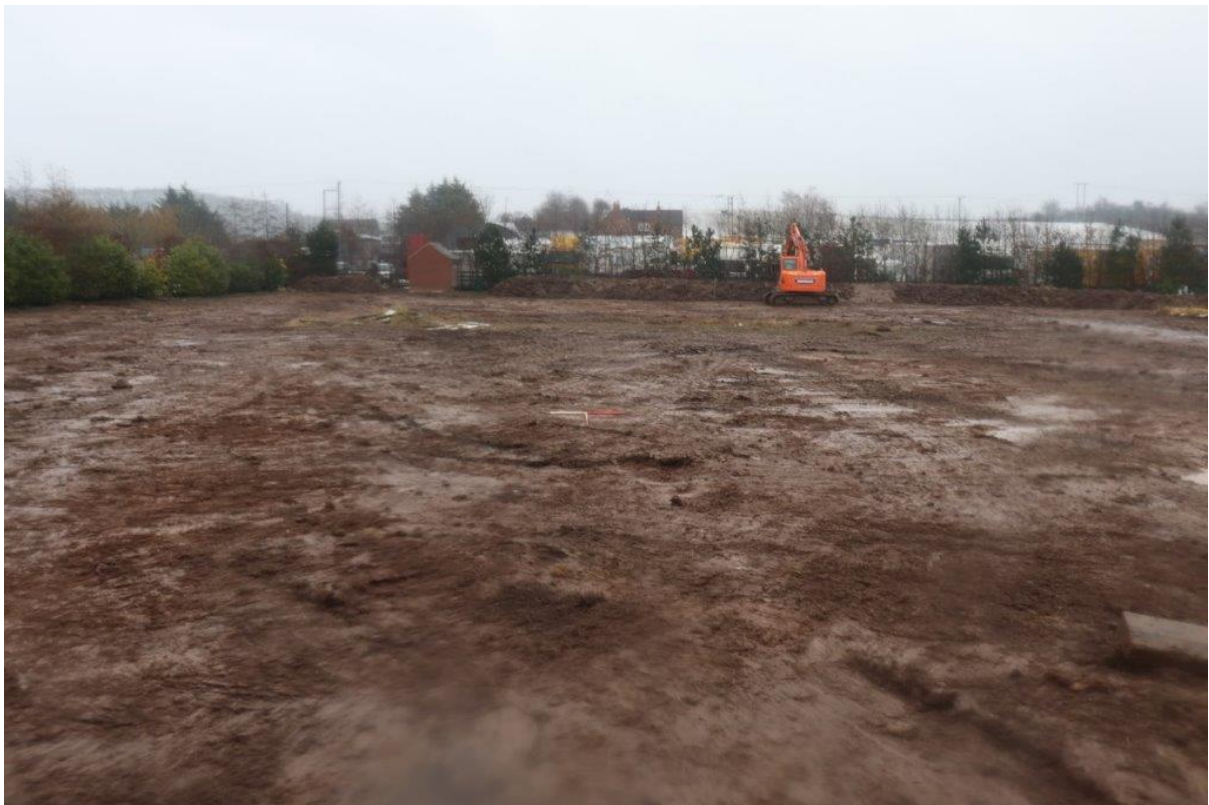
Plate 8: Topsoil strip complete at the centre of the site, looking east with 1m scales
