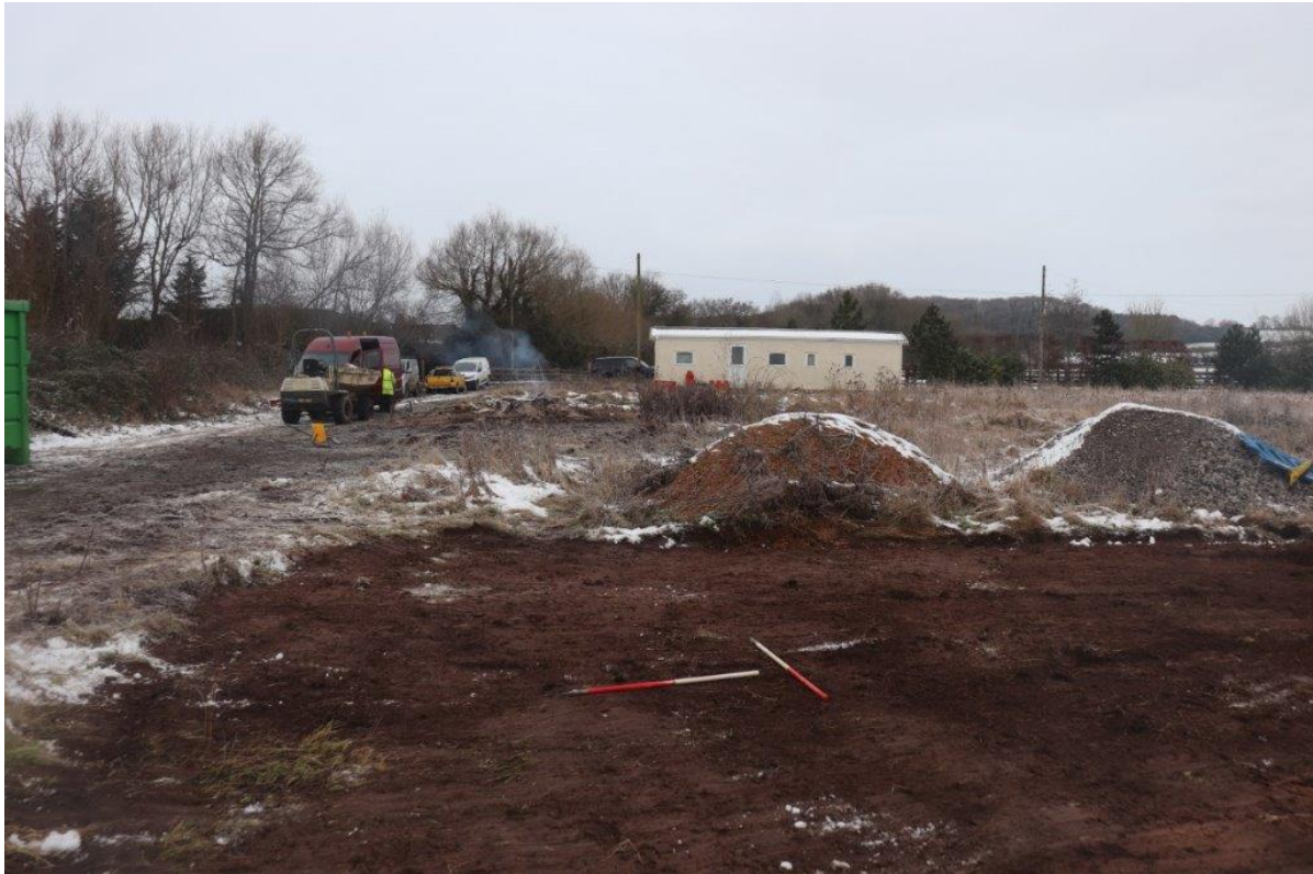
Plate 1: The site at the beginning of the works, showing the existing temporary road and static caravan, looking north with 1m scales
