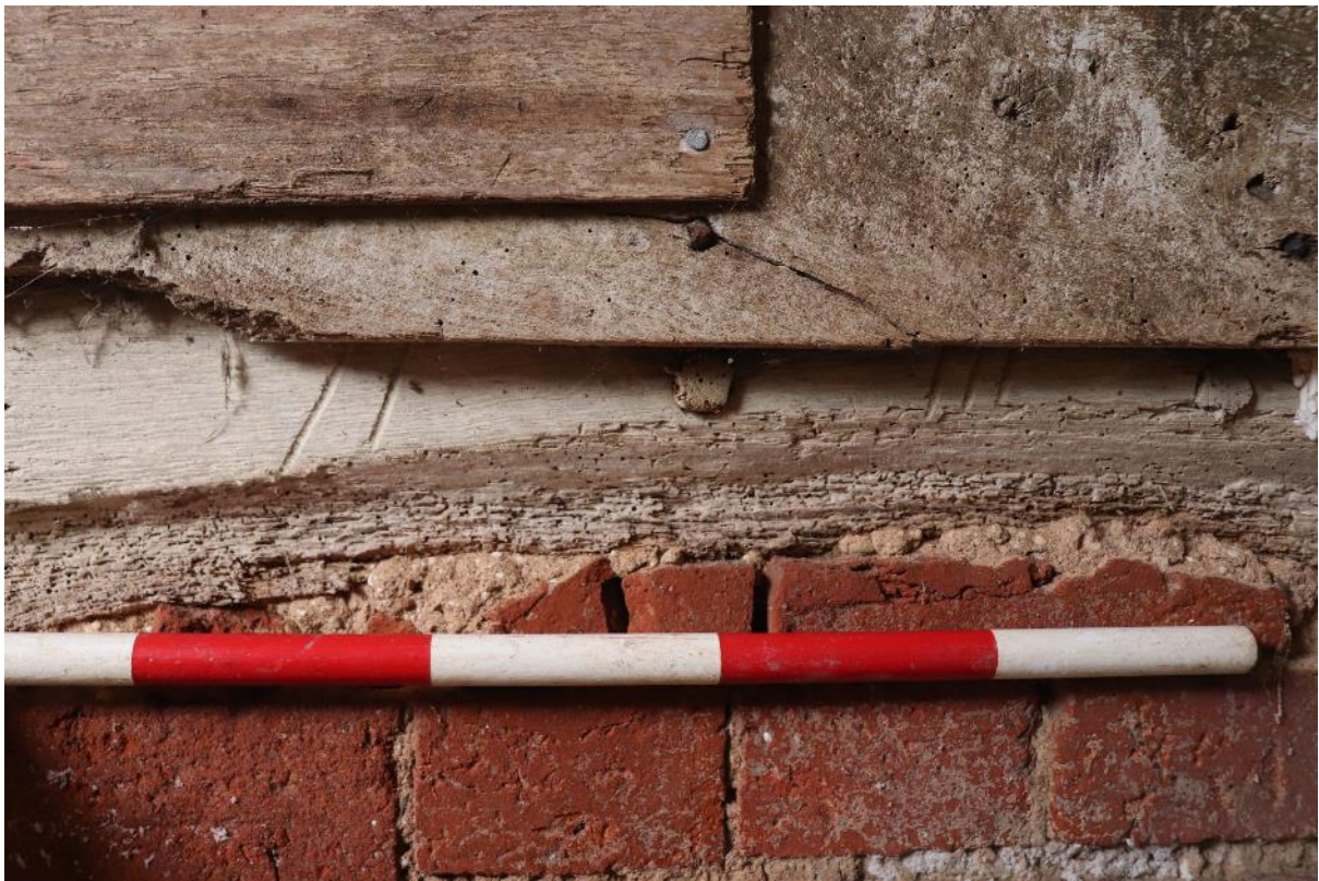
Plate 6 An example of the carpenters marks on the Phase 1 gable end, looking west, scale 0.5m
