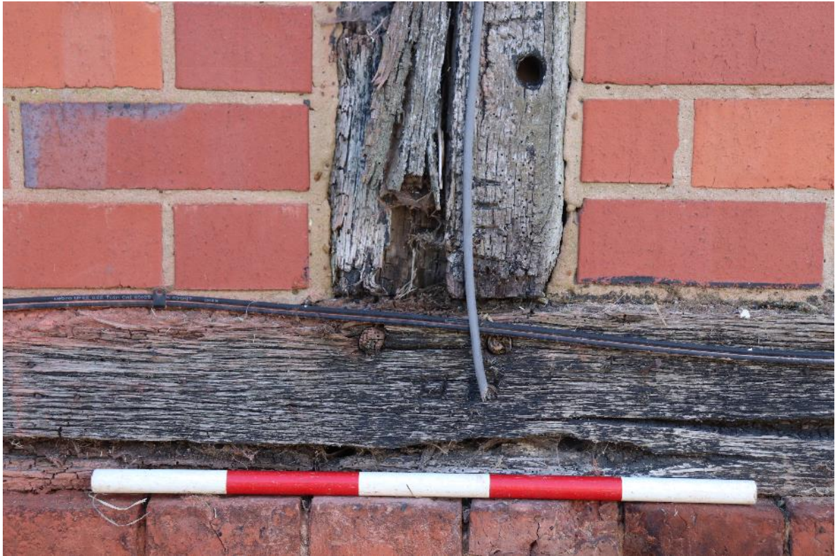
Plate 5 An example of the carpenters marks on the Phase 1 gable end, looking east, scale 0.5m
