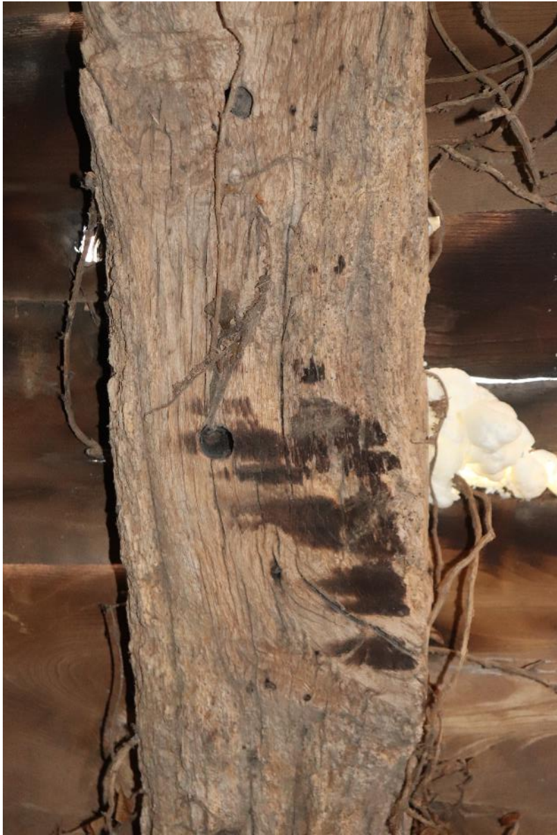
Plate 9 Burn marks on a Phase 1 reused timber, looking south
