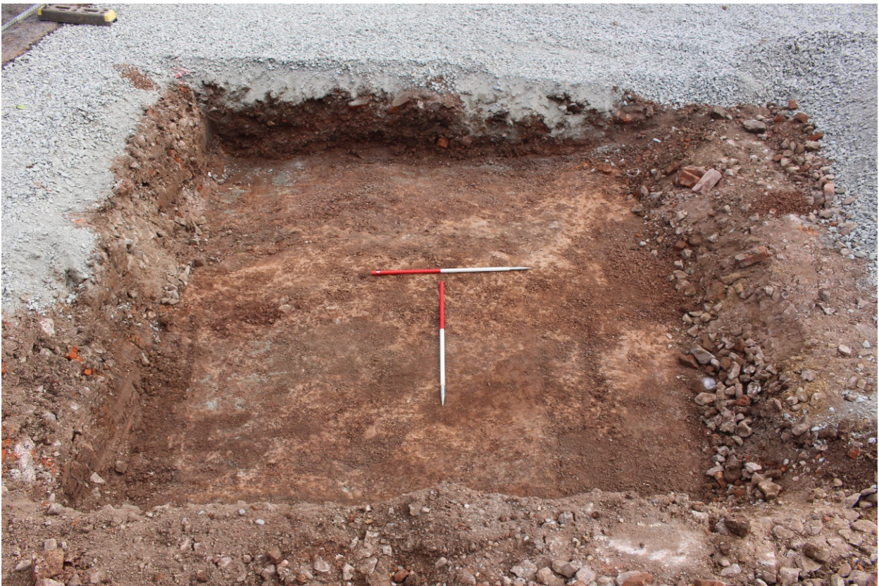
Plate 2: Trench 1 in area of recently demolished storage garages, facing north-east, 1m scales
