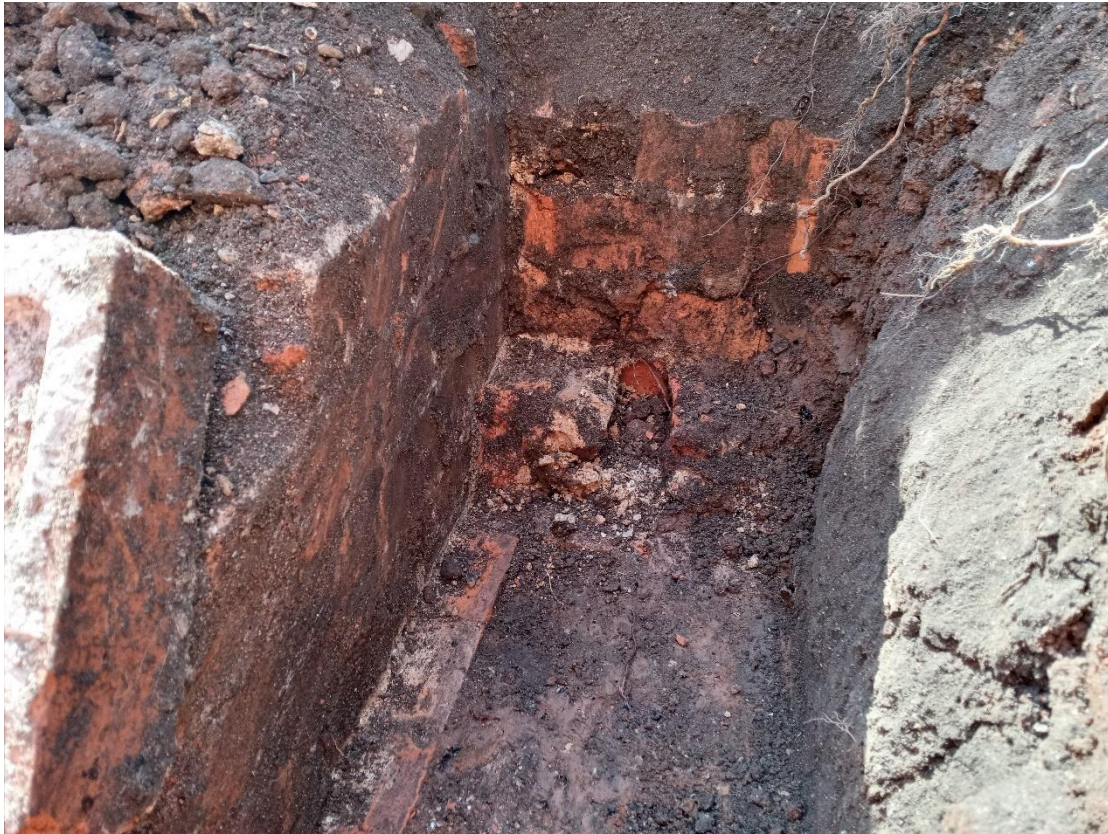
Plate 3: Junction of brick walls 103 and 104, forming the interior of the demolished 1840-1903 extension
