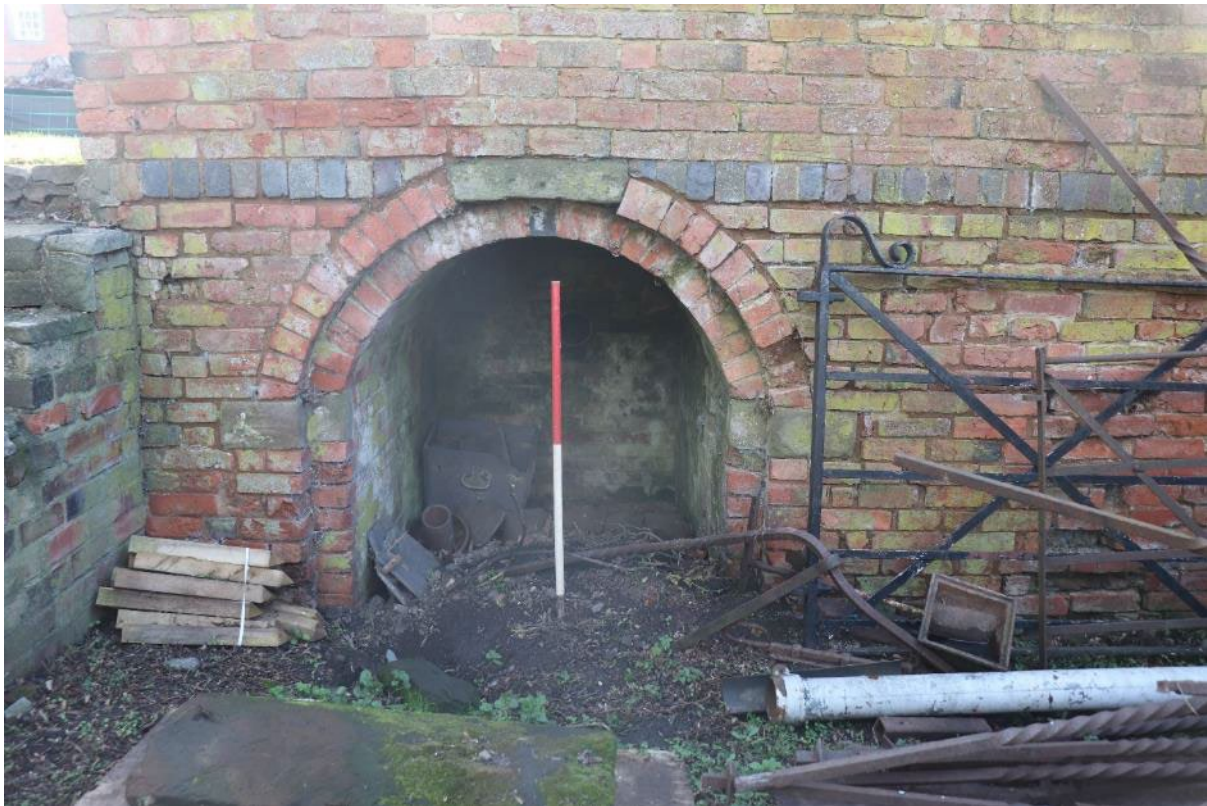
Plate 28: Outlet of brick culvert (503) at north-west edge of Lower Yard, view south-east; 1m scale
