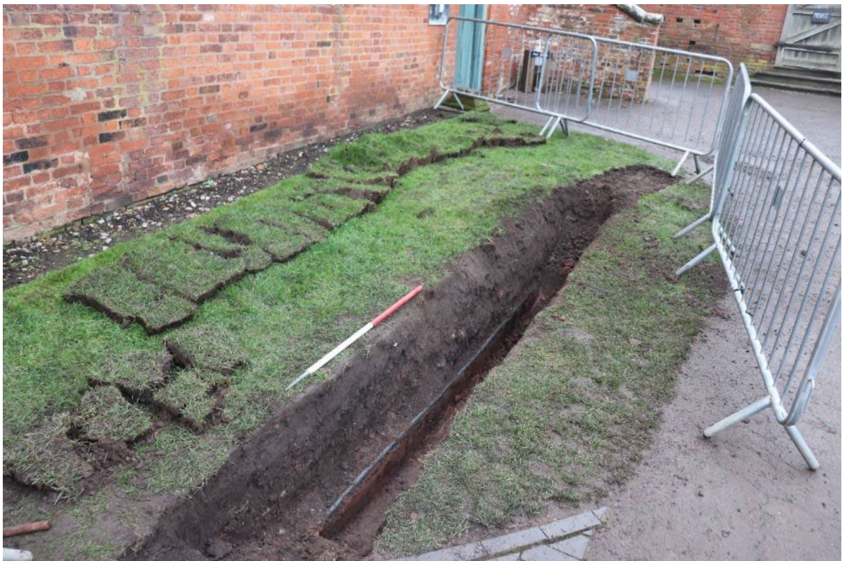
Plate 18: Trench 4 along north-east side of Service Yard with modern water pipe and disturbed ground, view east; 1m scale
