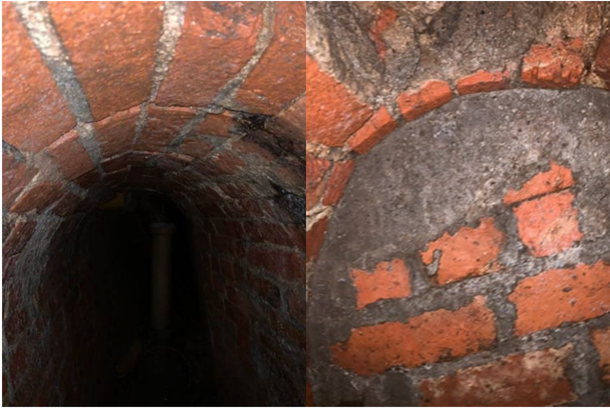
Plates 27a and b: Views inside brick culvert (503) from Trench 5, showing (a) pipes and intact condition to south-east; (b) bricked up to north-west, possibly due to modern drainage (502); no scale
