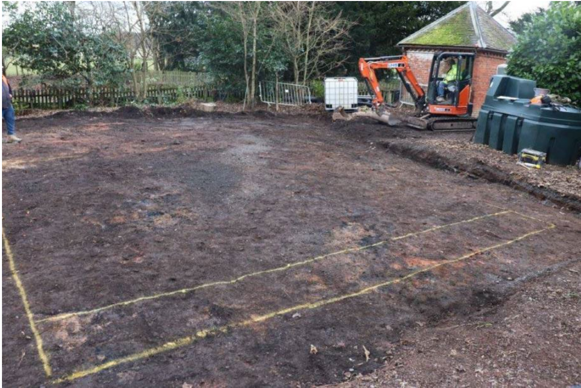
Plate 1: The site of the Biomass boiler (Trench 1) prior to excavating footings; view south-east towards game store, no scale
