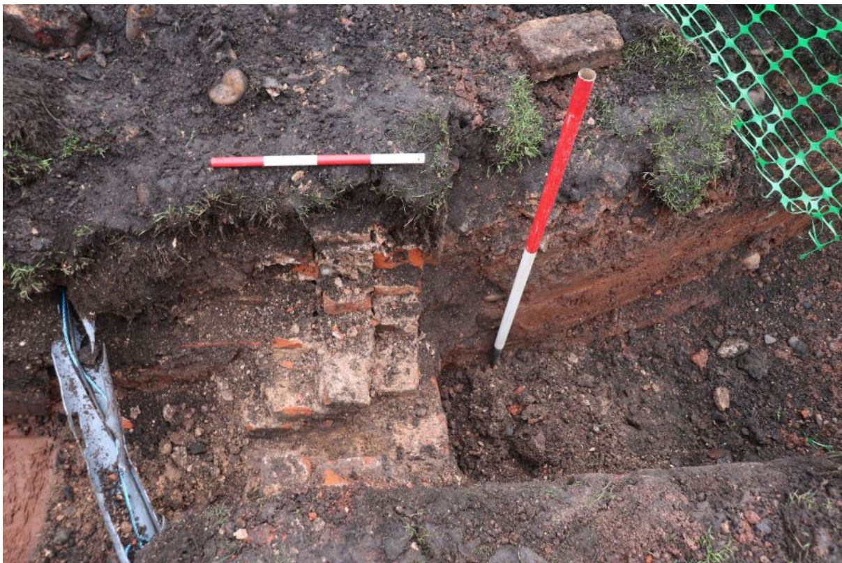
Plate 12: Trench 2, brick wall (204) at north-east corner of former stable block, partially removed, and drainage channel that ran into drain (209), heavily truncated by modern BT cable services; view south-east; 0.40m and 1m scales
