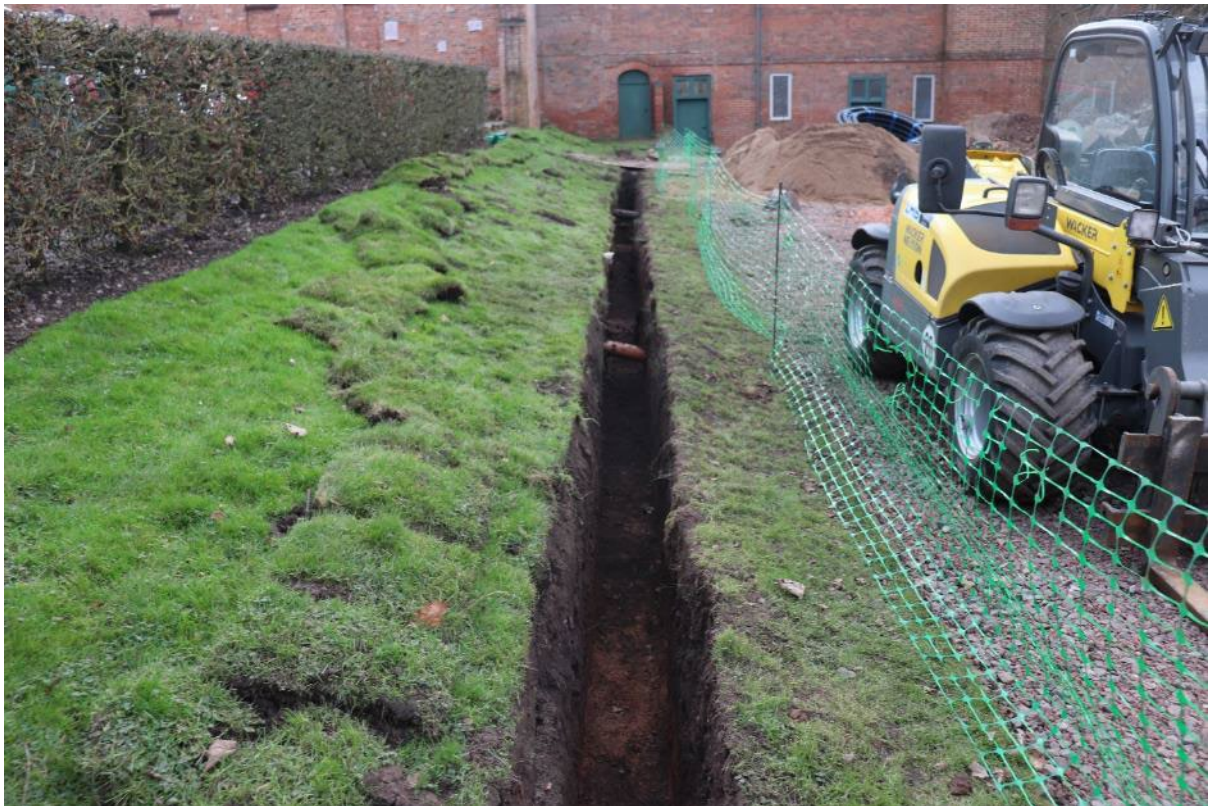
Plate 22: Trench 5 adjacent to hedge between Service yard and Lower Yard, view south-west; no scale
