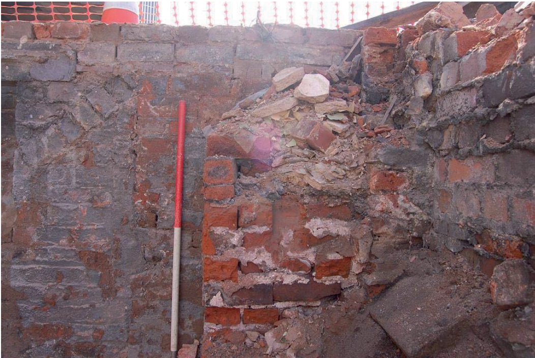
Plate 2, Wall and buttress 109 in south corner of North-West Range cellar, view southeast
