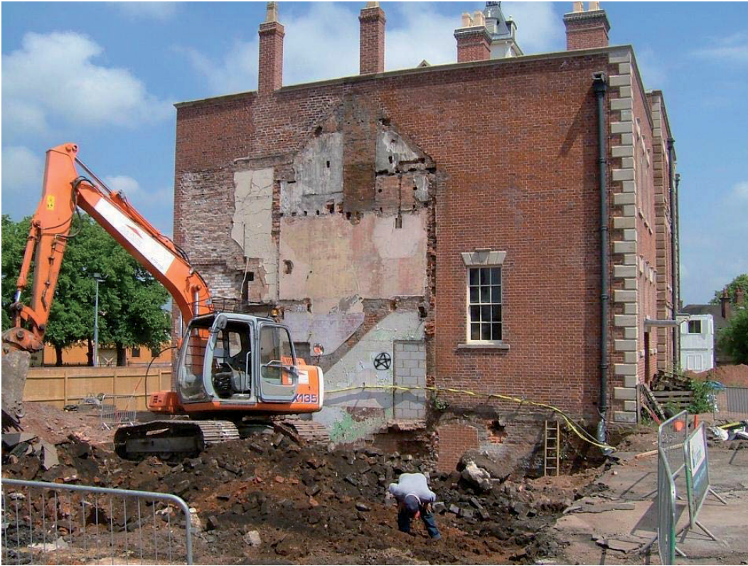
Plate 1, West elevation of West Range after demolition of North-West Range, view north northeast
