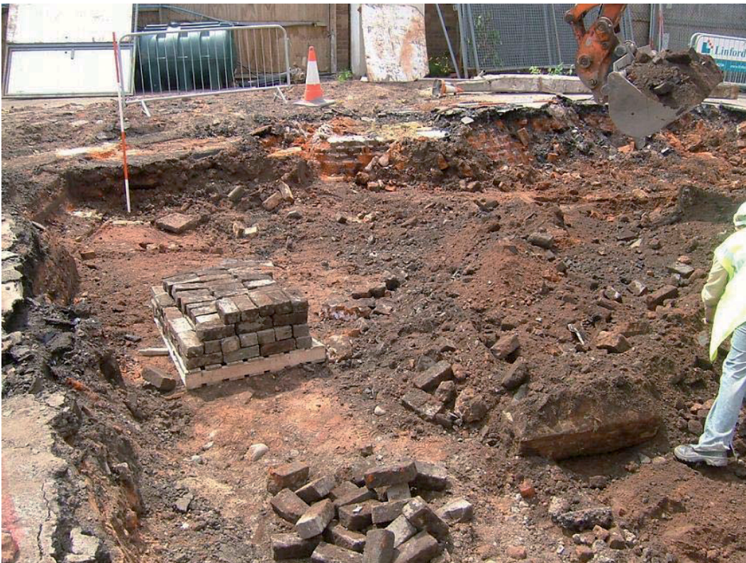
Plate 10, Brick buttress, 121, and excavation of footing for new Archive Store, view west
