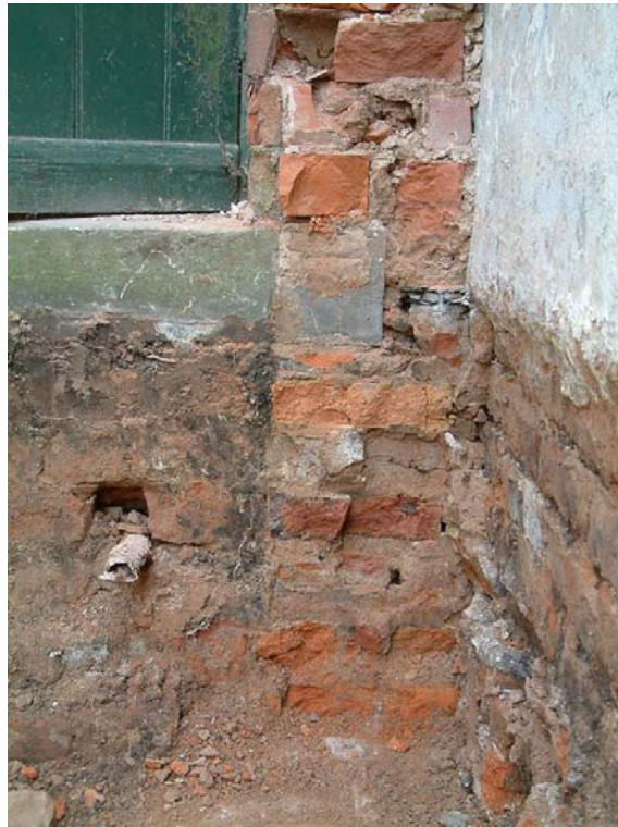
Plate 5, Area 2: Brick wall, 107, along west boundary below former School House lean-to, view south
