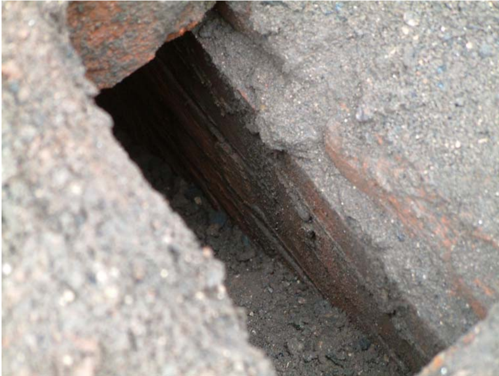
Plate 17, Area 8: south wall of north brick vault, 806, as broken through, view south-east
