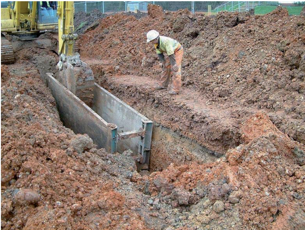
Plate 11: The excavation of the pipe trench in Trench 7, looking north northwest. The original buried dark topsoil (702) is clearly visible below made ground (701)
