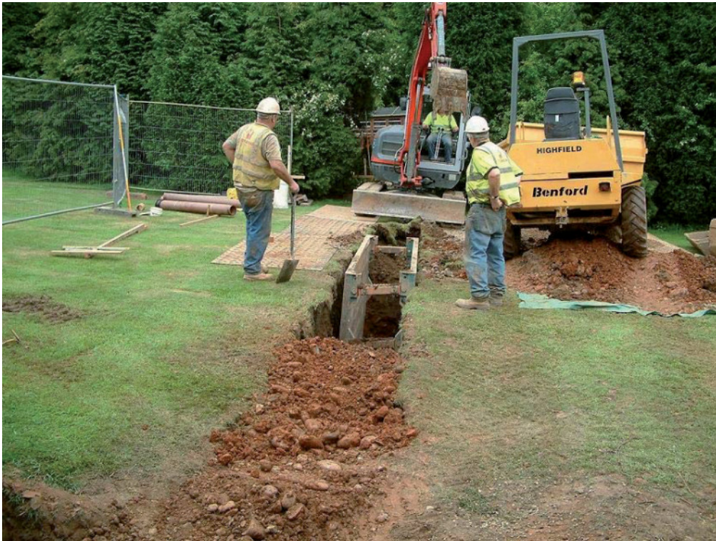
Plate 16: Trench 11, excavation of the pipe trench in the rear gardens to the southwest of Monument Lane
