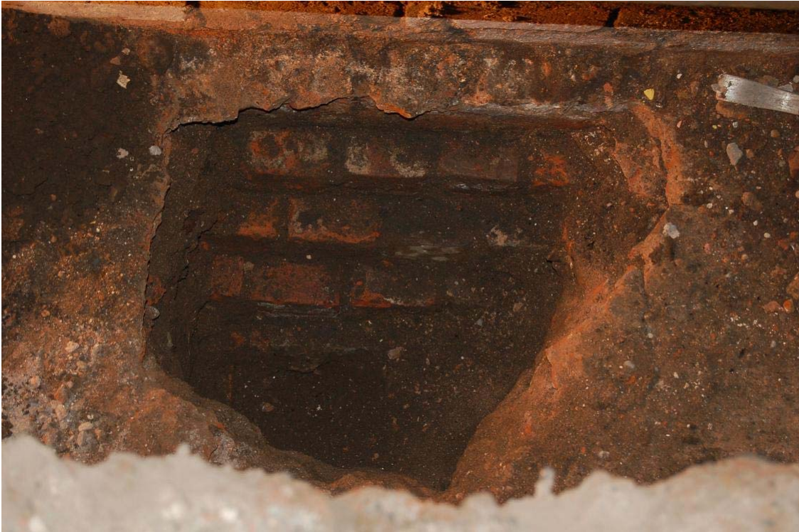
Plate 3 Sondage in test pit 1 showing stepped foundations of the east wall of the Scala Theatre
