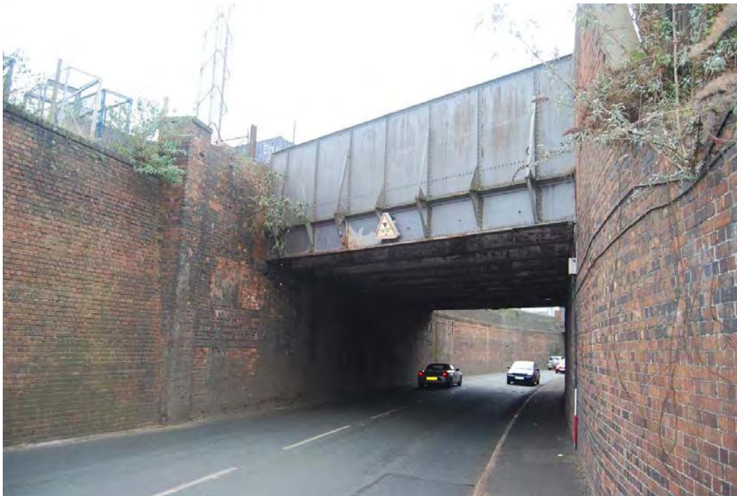
Plate 13. Showing the eastern side of the bridge from street level. Looking west.
