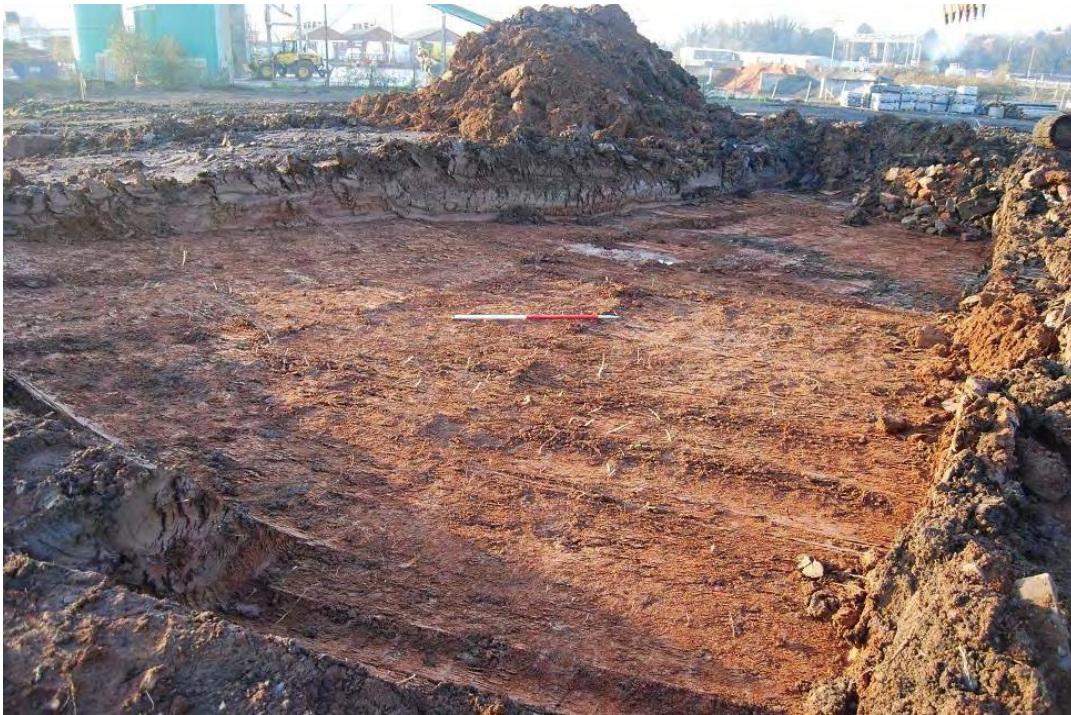
Plate 1. Stripping of the access road next to Tolladine road. Modern overburden deposit 100 can be seen overlying natural deposit 101. Looking northwest.
