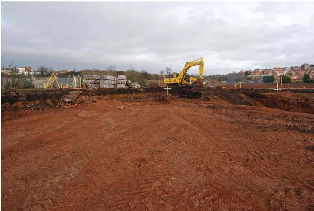
Plate 4. Southern area of access road after stripping. Modern overburden 102 can be seen overlying natural deposit 101.
