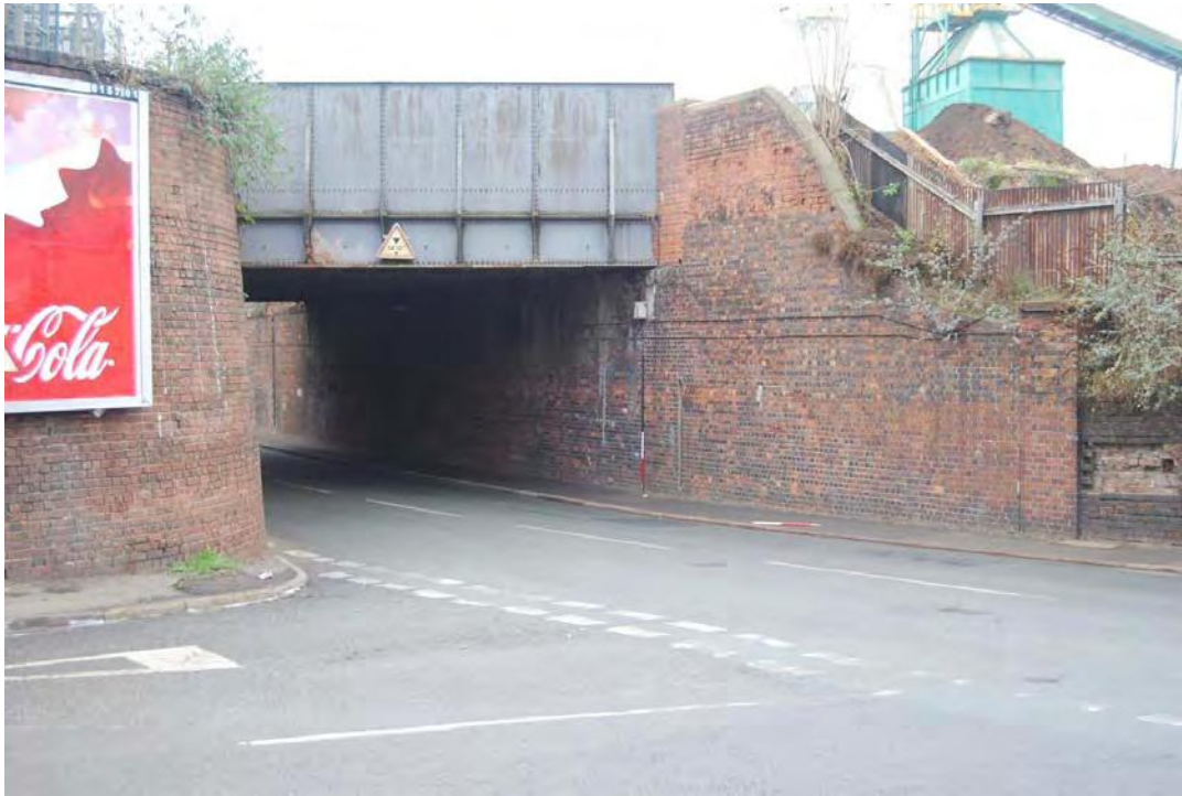
Plate 12. The eastern side of the bridge and retaining wall (which is to be removed). Looking northwest.
