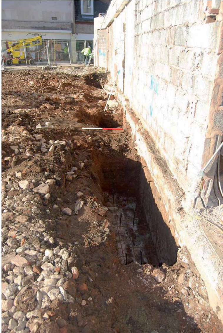
Plate 3. Area 2: Showing bases excavated to the northeast of the site onto an existing concrete footing
