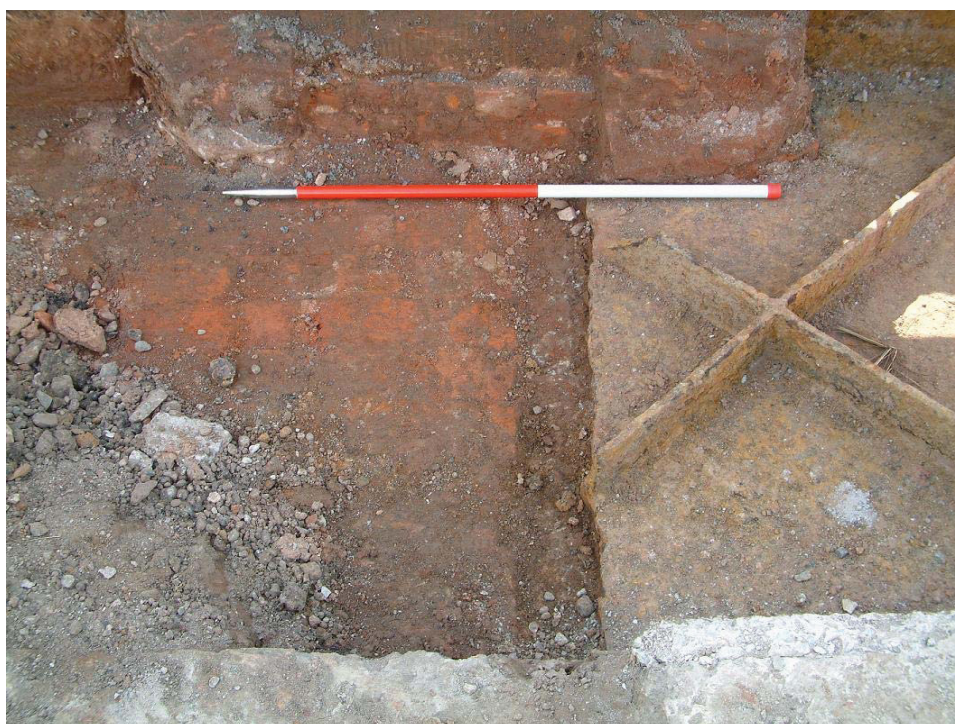
Plate 2, Edge of metal plate 1022 and brickwork 1013 adjacent to Trench 1 in southwest footpath, view southeast
