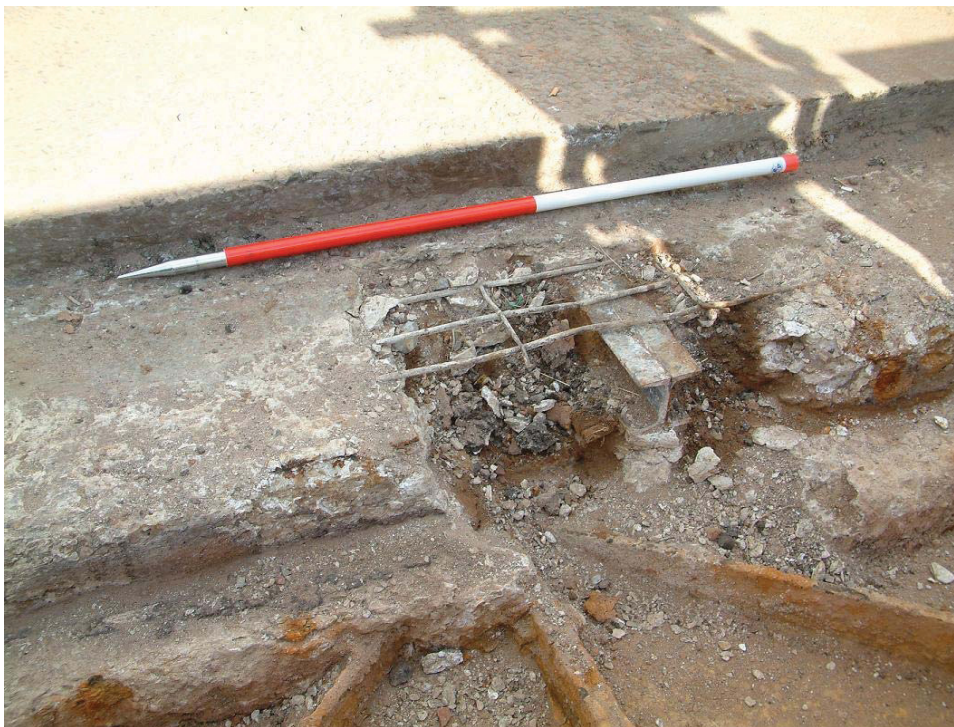
Plate 10, steel reinforced concrete and iron rail adjacent to southwest footpath on southwest side of bridge, view northwest
