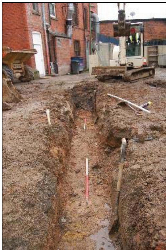
Plate 7 Central trench after excavation showing building rubble and modern service disturbance above the natural clay
