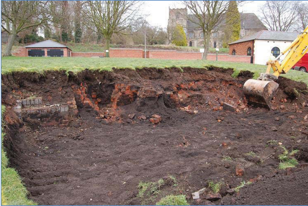
Plate 3 Trench 1 during excavation showing the partially demolished 20 th Century wall (103) looking northwest towards St Mary's church
