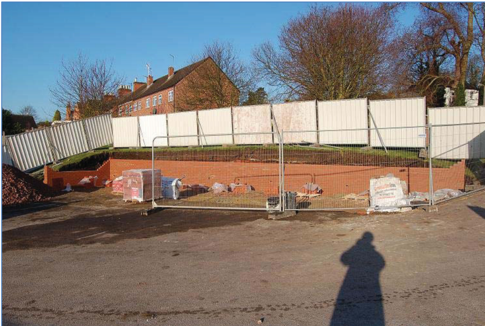
Plate 6 Trench 1 completed with hardcore surface and retaining wall being constructed looking north
