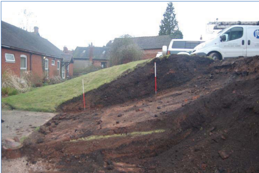
Plate 16 Trench 3 area for steps after excavation showing made ground (302) and natural (303 + 304) looking southeast
