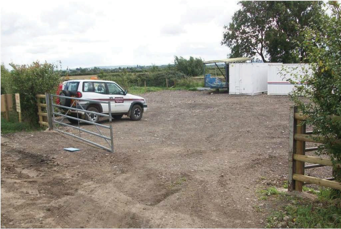
Plate 10 General view south-east of Site Compound after area reduced and stone laid
