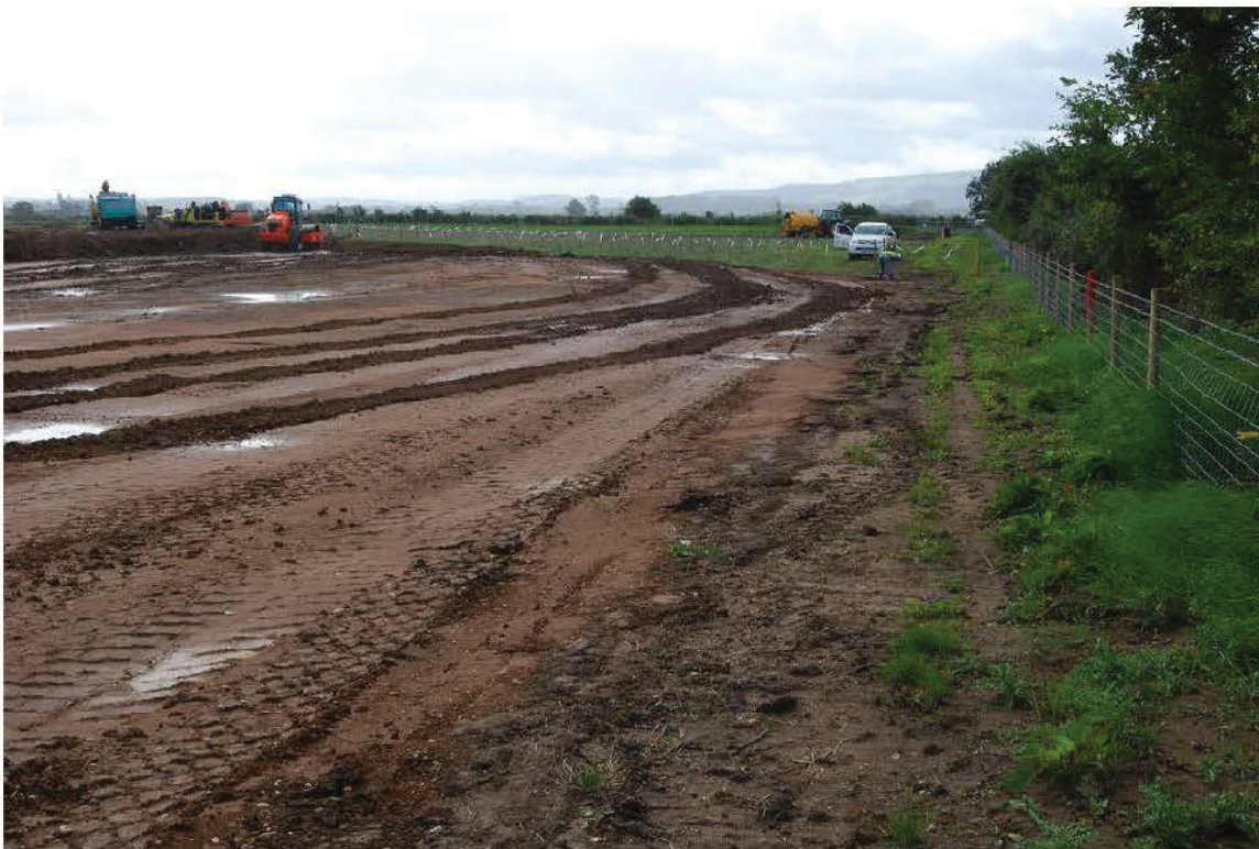
Plate 9 General view south of ground reduction within north-east corner of Scheduled Ancient Monument, north of Access Road, after excavation and replacement of material
