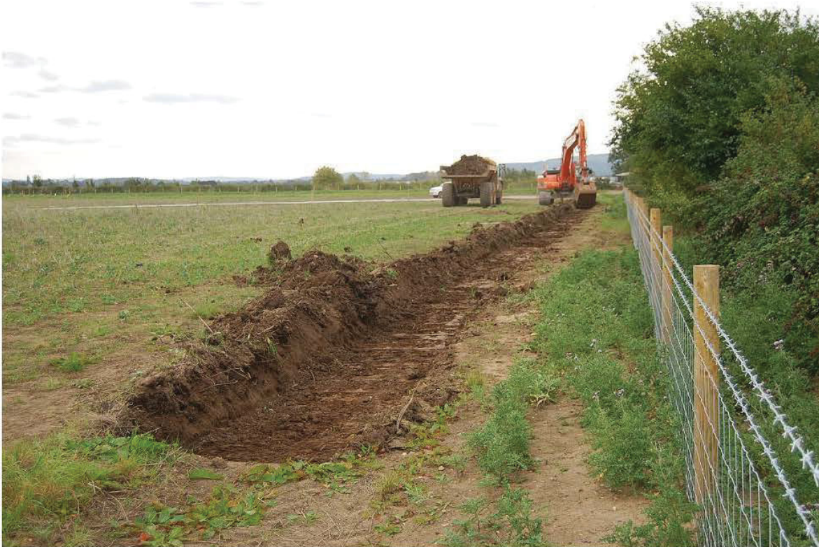
Plate 7 Stripping of the north to south aligned access road within the Scheduled Ancient Monument, view south
