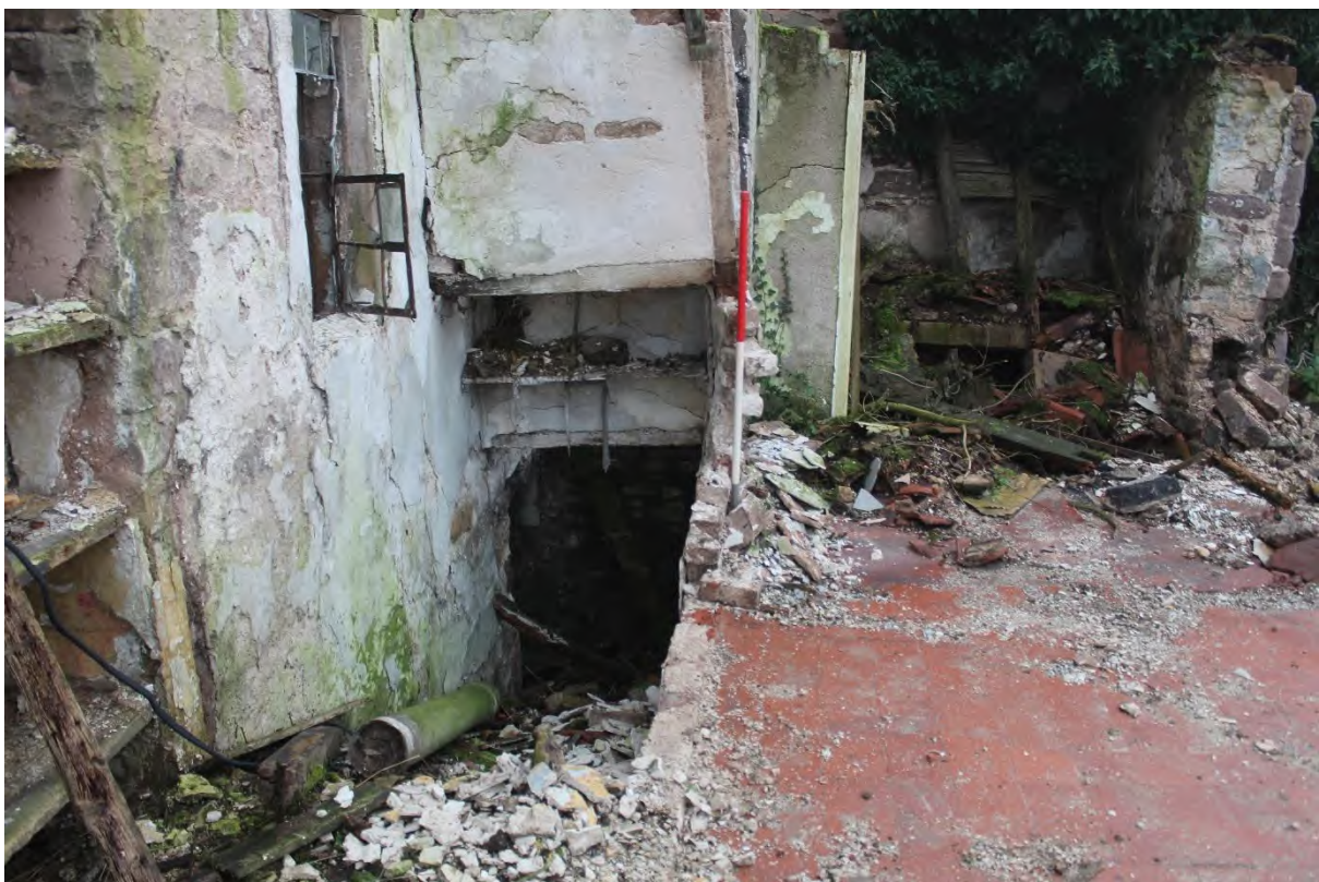
Plate 34. Farmhouse: Ground Floor Room 10 Entrance to Cellar after partial demolition (IMG_0104). Facing West.
