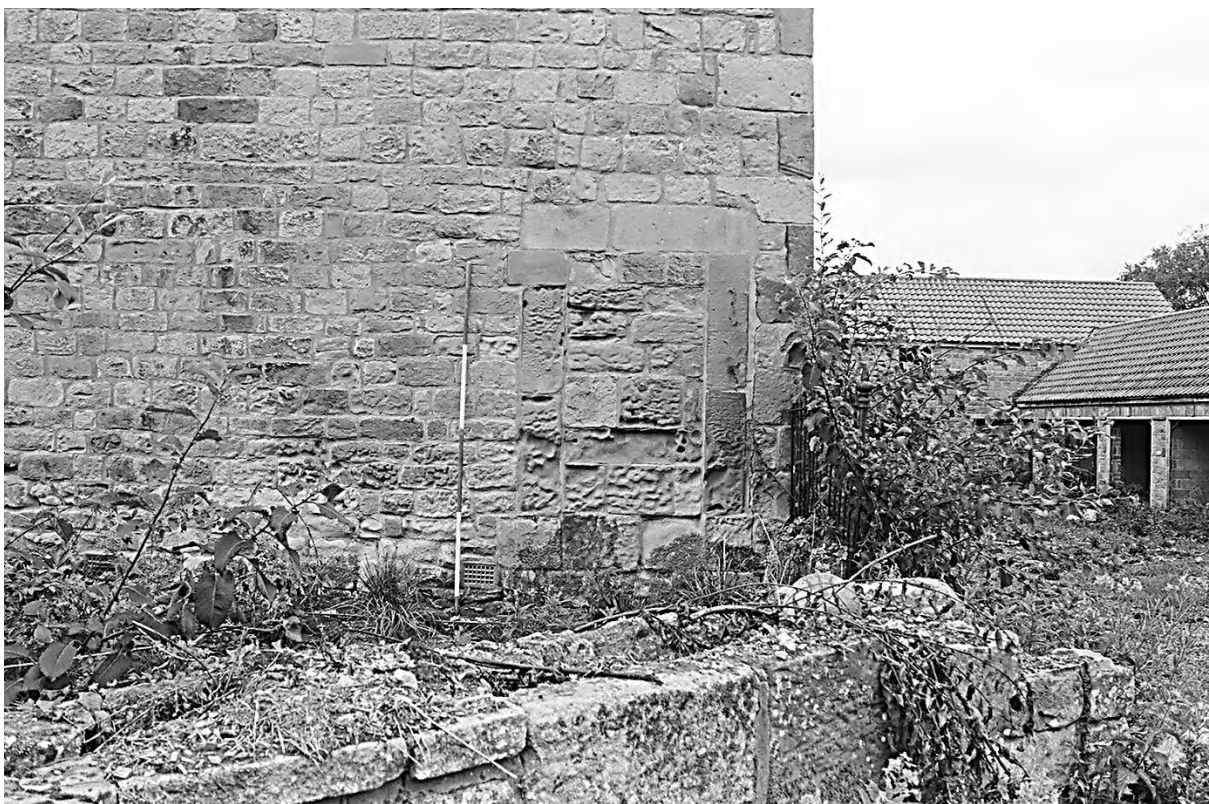
Plate 24. Farmhouse: South Elevation Blocked Door (Film 4/9). Facing North.
