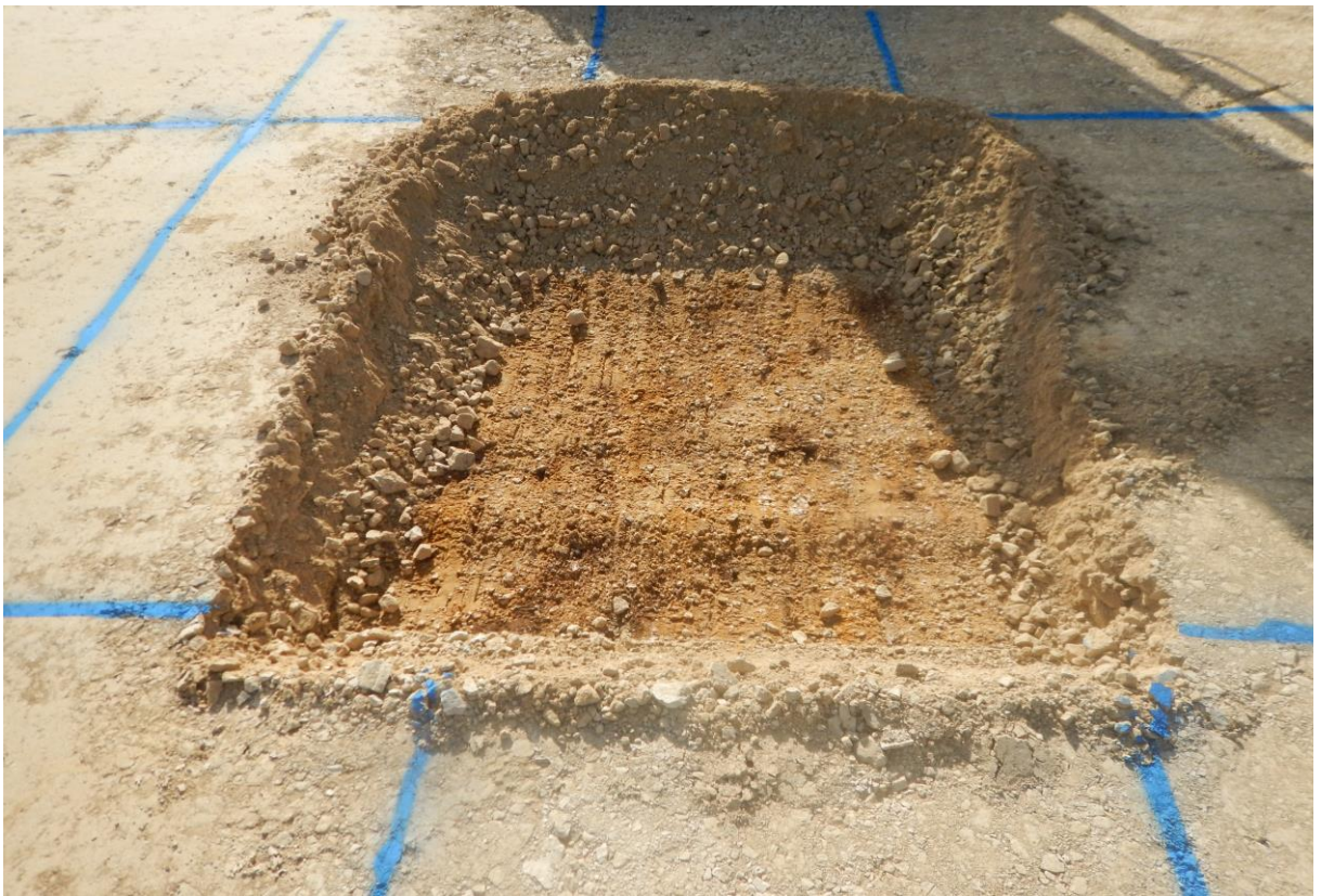
Plate 7. Typical Stanchion Base Showing Natural Deposits
