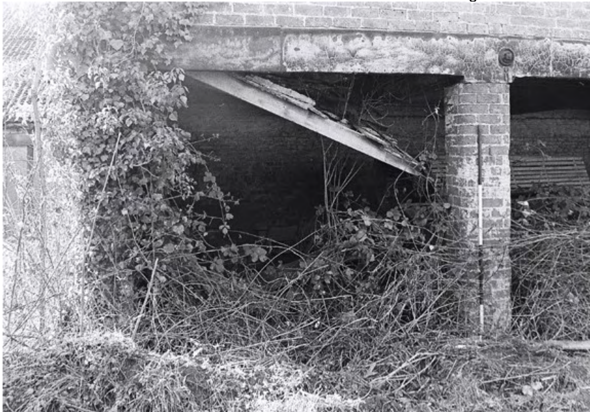
Plate 8. Cart Shed Exterior: Collapsed Floor. Facing West.
