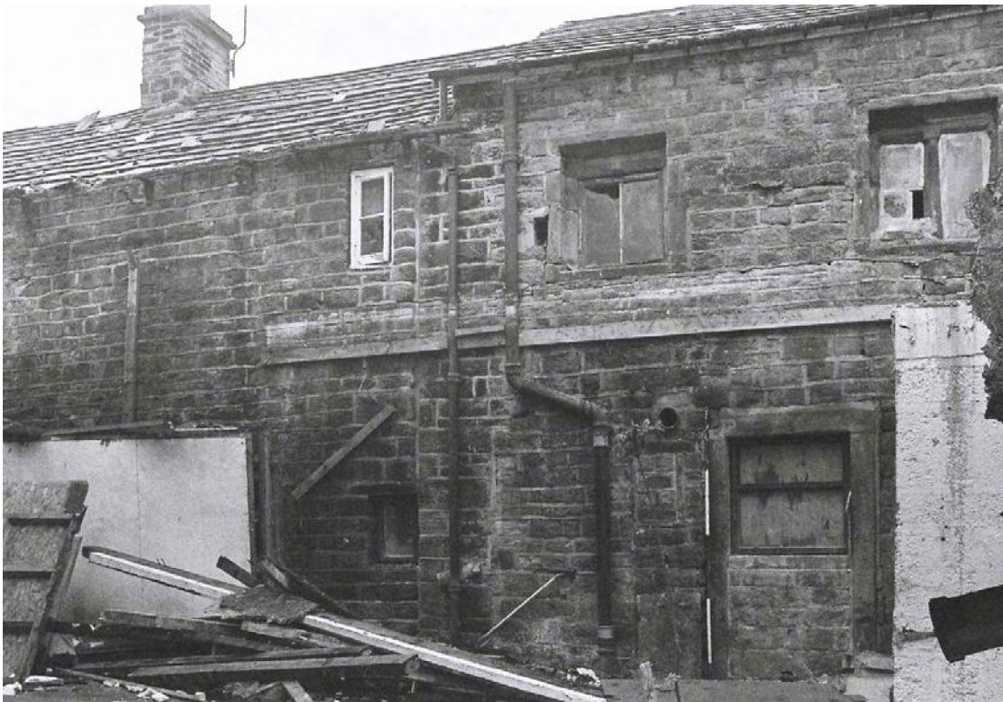
Plate 15. Shaw House Farm: Barn and Cottage Exterior (after demolition of Lean-to). Facing South.
