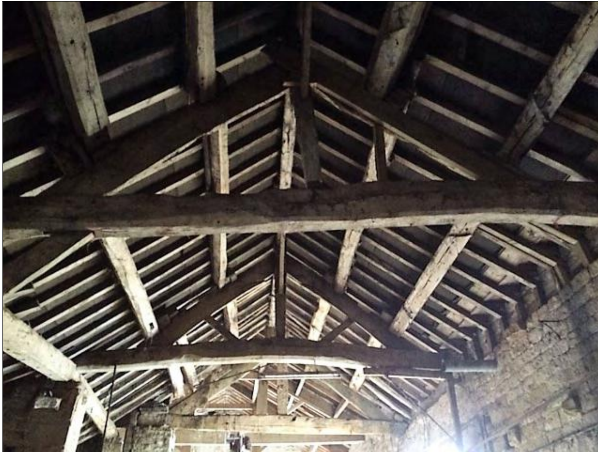
Figure 4: Barn roof with truss 1 in the foreground, photograph taken from the west
