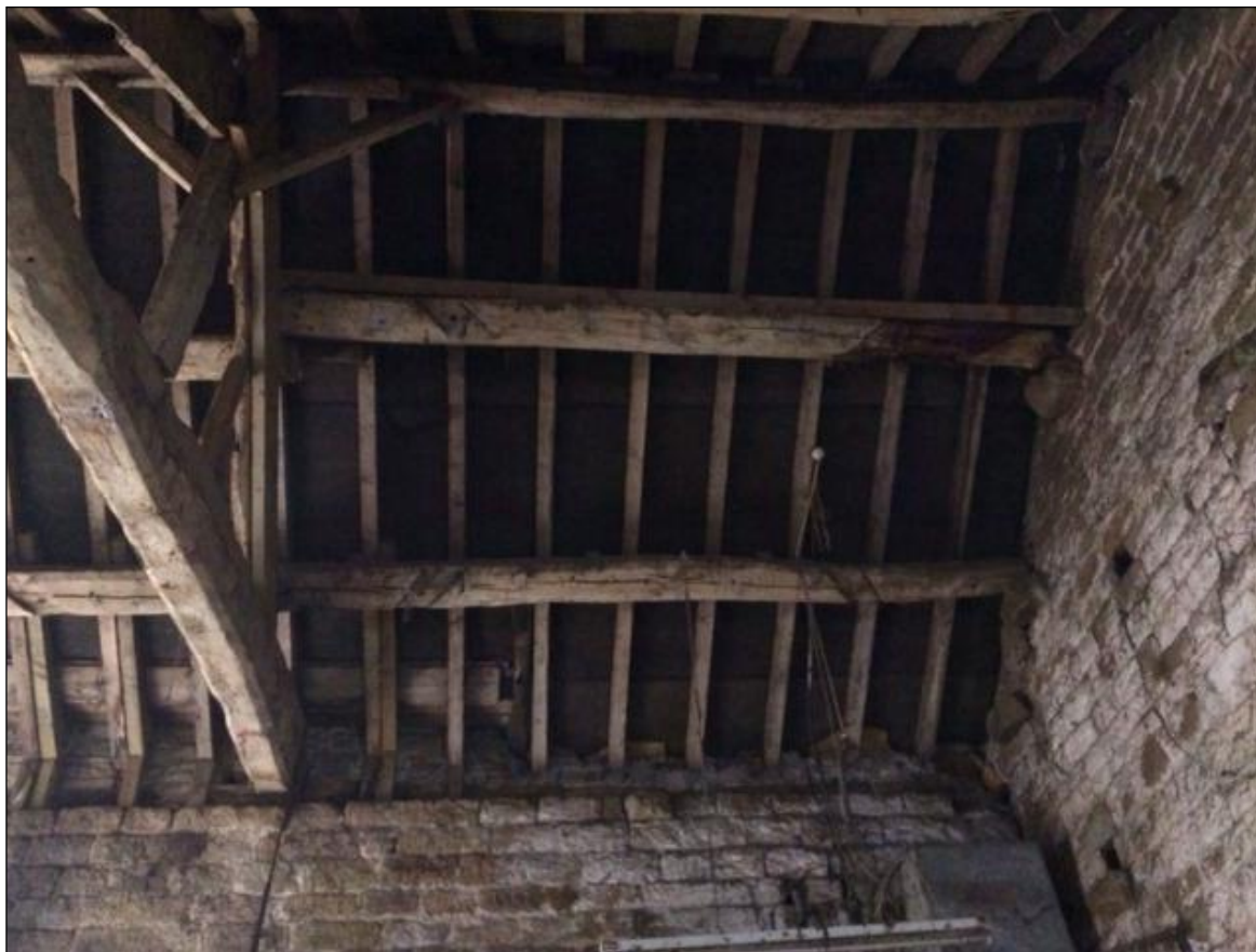
Figure 6: Bay 1 (south side), showing the purlins with redundant mortices, photograph taken from the north
