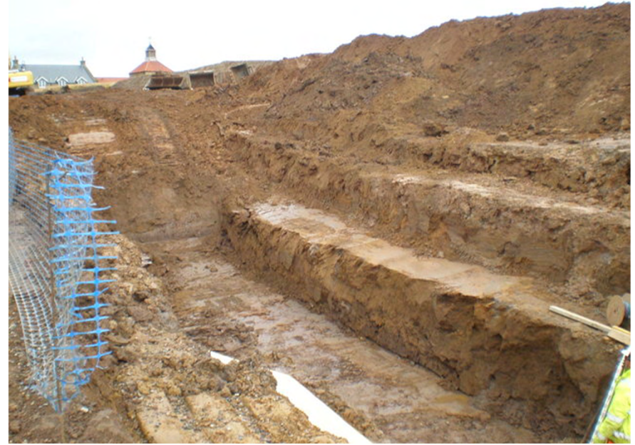
Plate 2. Section through Pipe Line Excavation Trench (Northern end of WwTW). Facing North-east.
