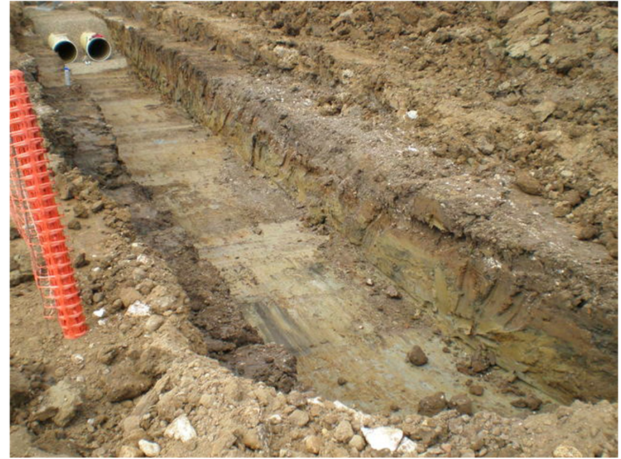
Plate 4. Section through Pipe Line Excavation Trench (Central Area of WwTW). Facing North.
