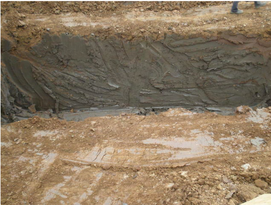
Plate 5. Section through Pine Line Excavation Trench. (Southern end of WwTW). Facing North.
