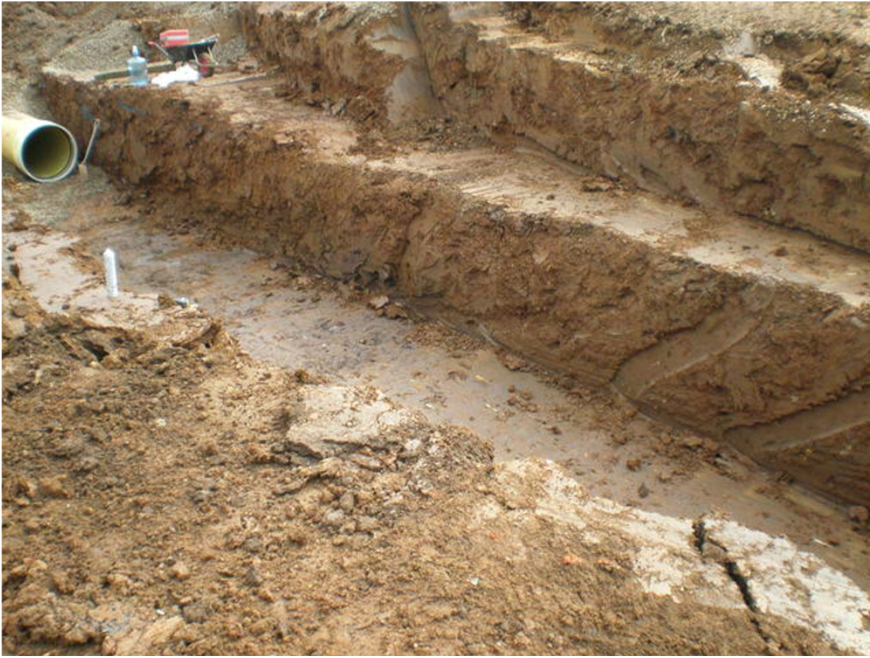
Plate 3. Section through Pipe Line Excavation Trench (Central Area of WwTW). Facing North-west.
