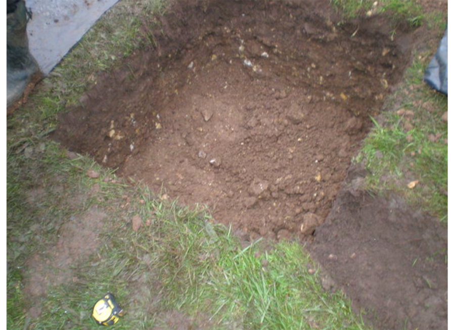
Plate 4. Soakaway Pit. Facing North-east.
