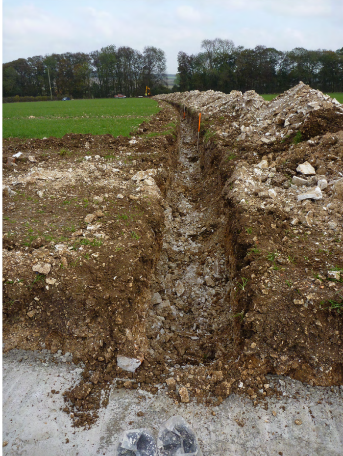
Plate 13. Turbine 2 section of cable run - north facing section. Facing South.
