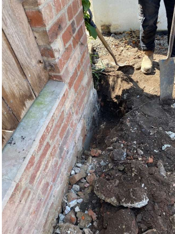
Plate 3: Excavation of test pit to expose the garage foundation depth. Facing south.
