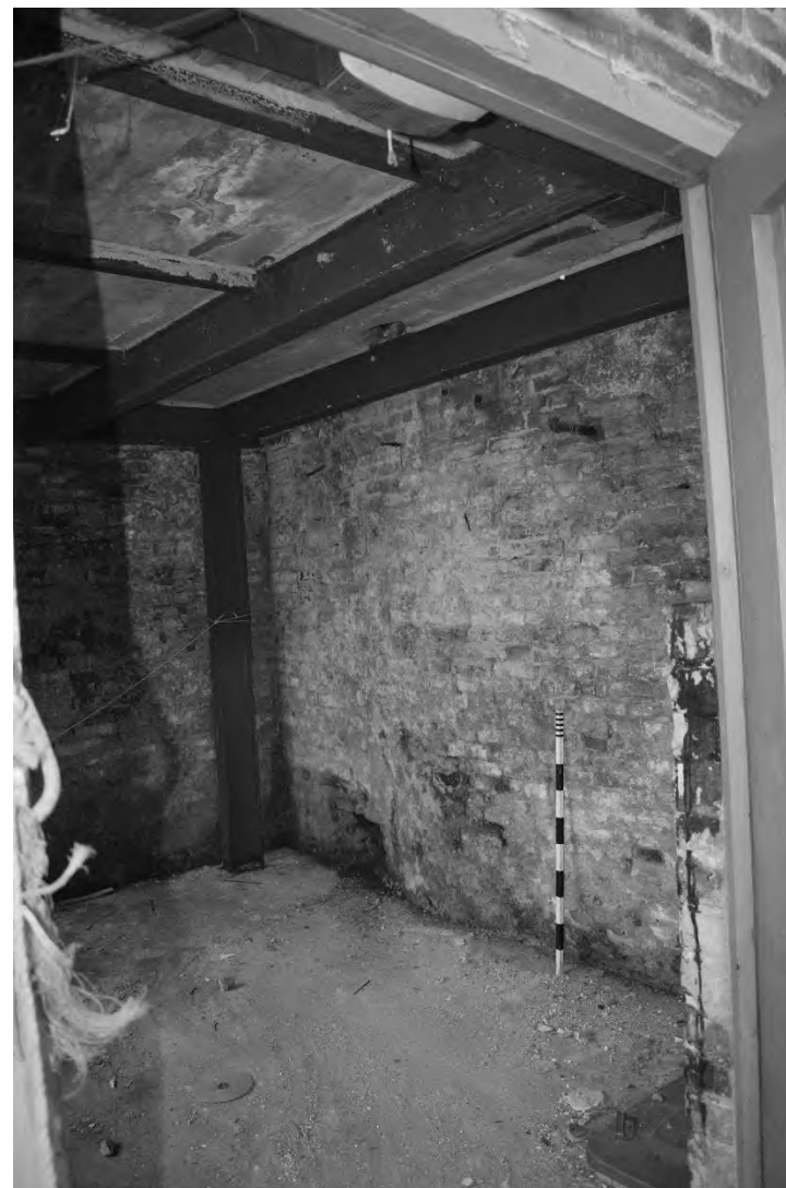
Plate 44. Interior First Floor Store: bowing wall & structural steelwork (DSC_0647). Facing North-east.
