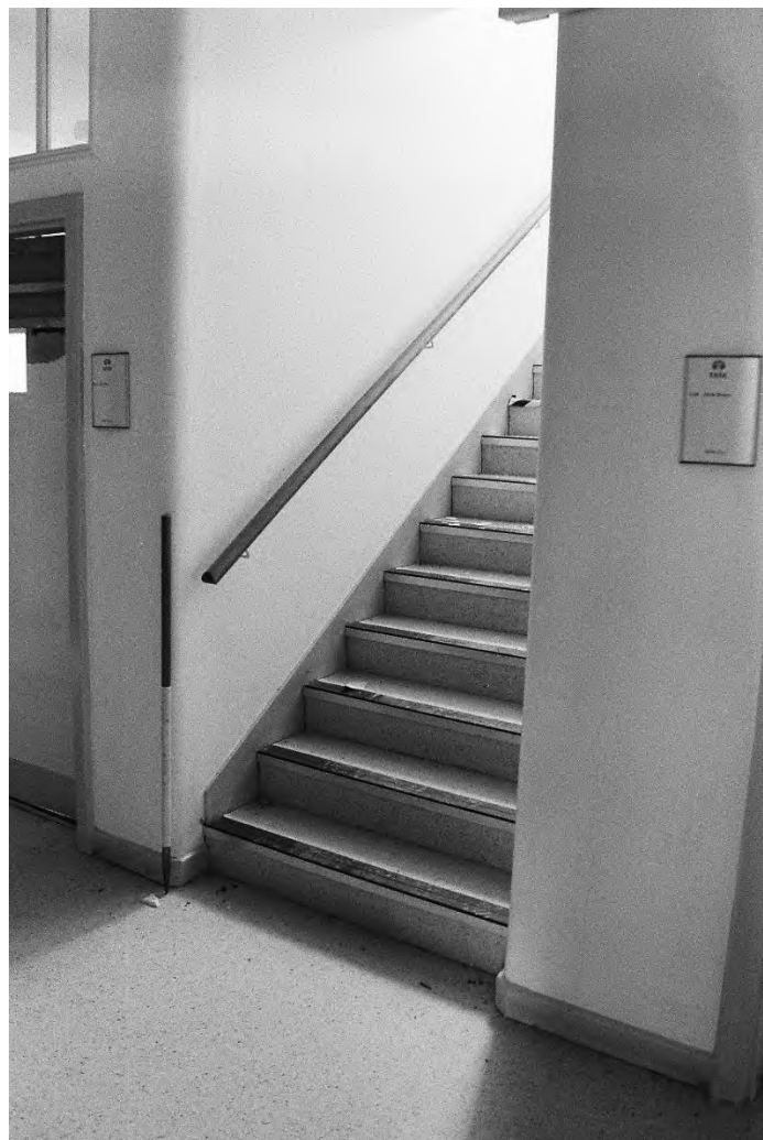
Plate 90. Block C: Interior First Floor Stairs to Room C193 (Swinden11_26). Facing South-west.
