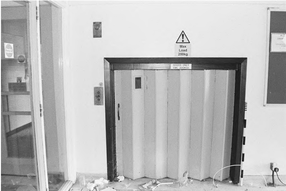
Plate 125. Block H: Interior Ground Floor Goods Lift (Swinden3_16). Facing West.
