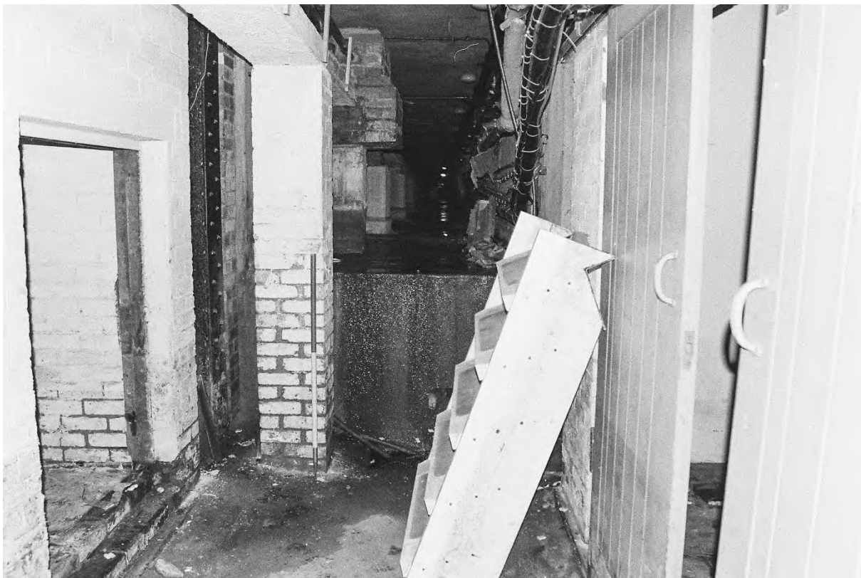
Plate 126. Block H: Interior Basement Duct (Swinden7_24). Facing South.
