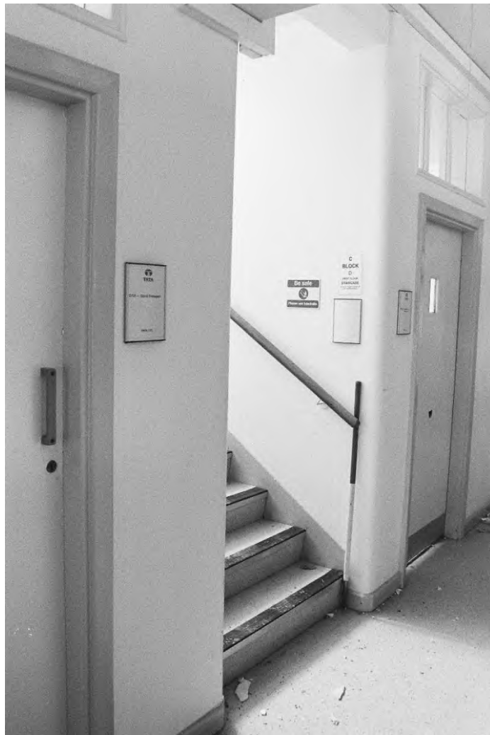
Plate 91. Block C: Interior First Floor Stairs to Room C192 (Swinden11_31). Facing North-west.
