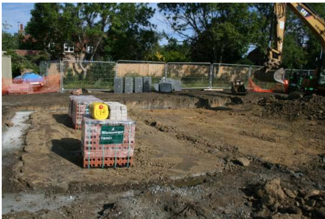
Fig. 8: Land at Burtenshaw Lane, Market Street, Hailsham: Photograph of house foundation excavation
