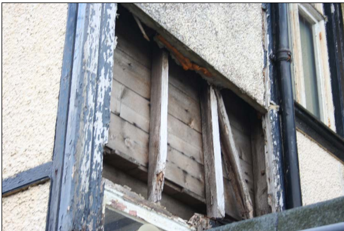
Fig. 15: 1 Cricketfield Road, Seaford: External view of construction showing missing concrete panel
