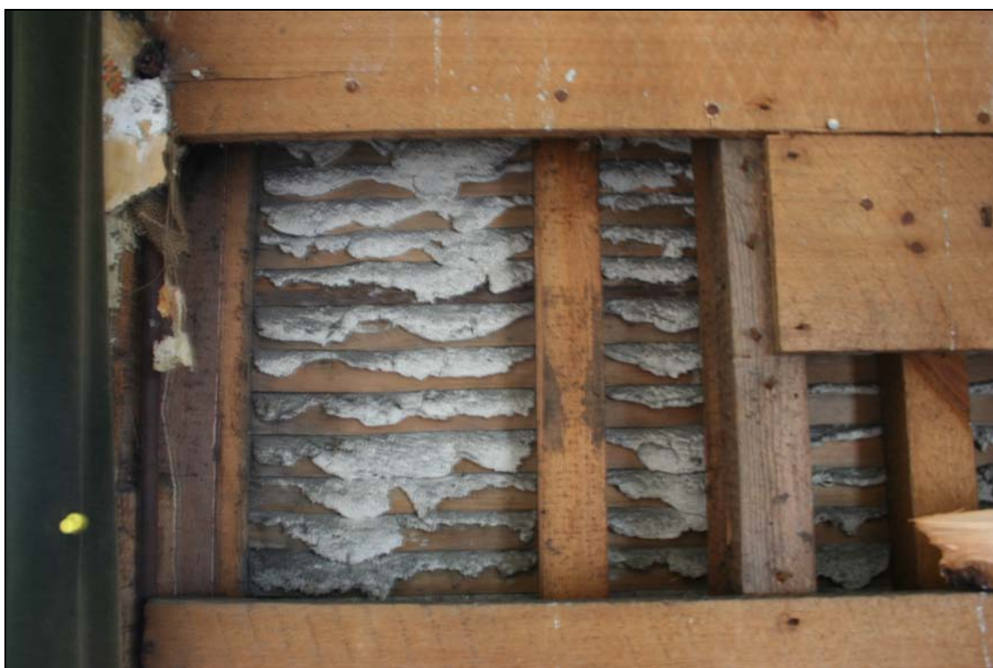
Fig. 16: 1 Cricketfield Road, Seaford: Interior view of construction showing laths and wooden framework, and wooden plank walls
