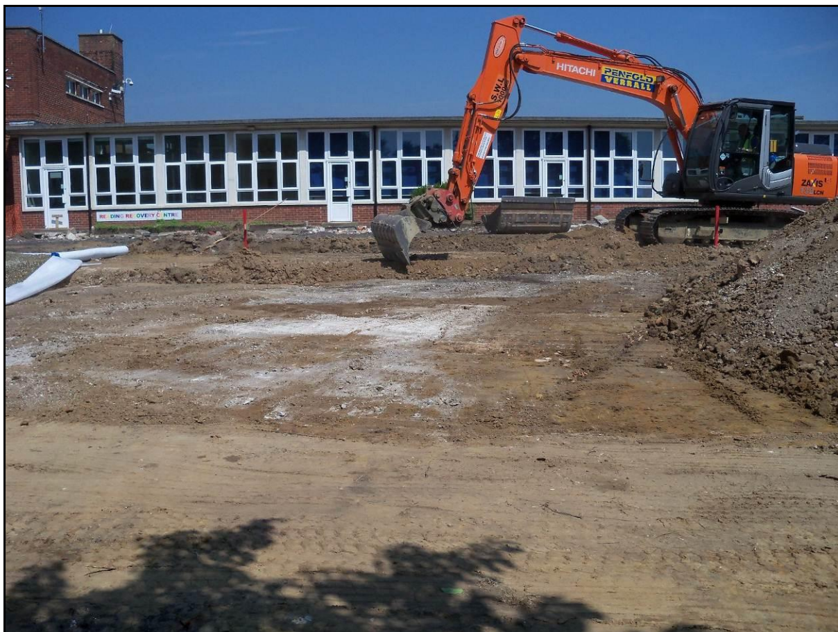
Plate 5: Highfield Junior School, Eastbourne: West side of site after ground reduction, looking north
