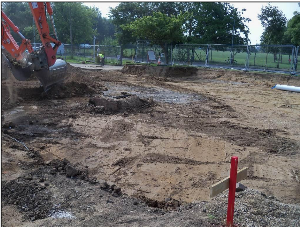
Plate 4: Highfield Junior School, Eastbourne: Southwest corner of site after ground reduction, looking southeast
