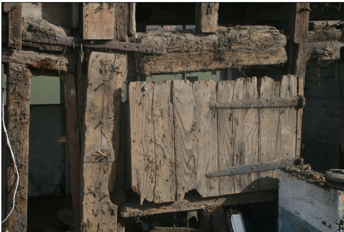
Fig. 16: Crown View, Horsted Keynes: Shutter revealed in south wall during demolition
