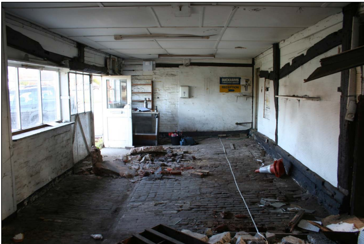
Fig. 11: Crown View, Horsted Keynes: Inside the stable building showing brick floor & south wall on right side
