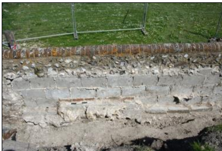
Plate 2: Alciston Church: Modern repairs to wall
