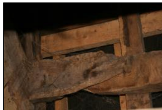
Plate 33: Joint in Purlin South Side Bay 1
