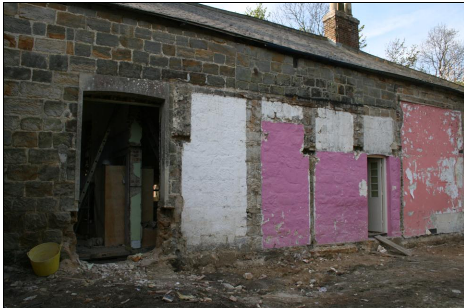
Fig. 8: Ore Place Farmhouse: North wall of Farmhouse showing original entrance noted by the change in the stonework to the right of the large doorway to the far side of the small doorway
