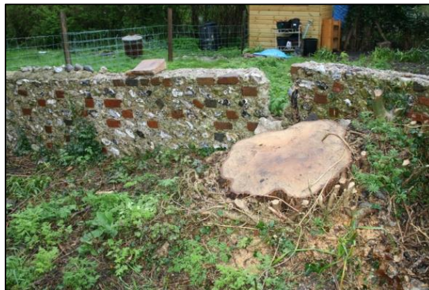
Plate 7: Tree Damage to Wall
