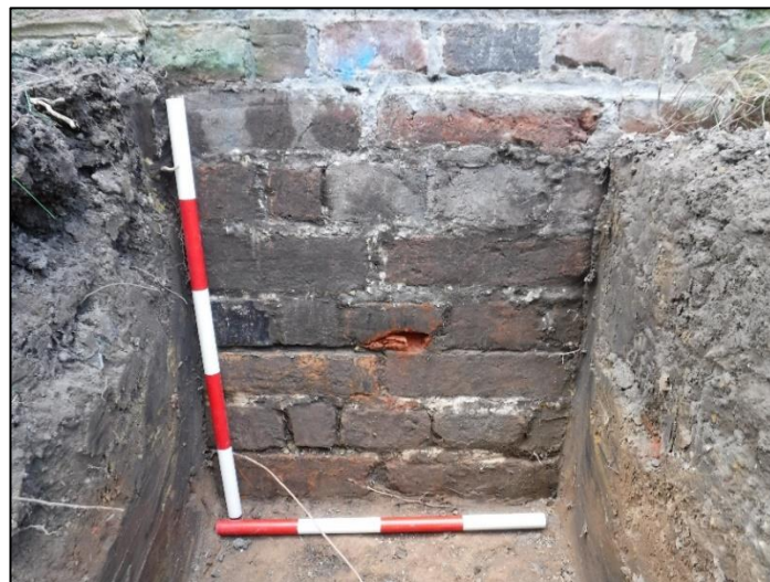
Plate 3: East-facing section of foundation wall to existing building (Context 004 ). 0.4m and 0.5m scale.
