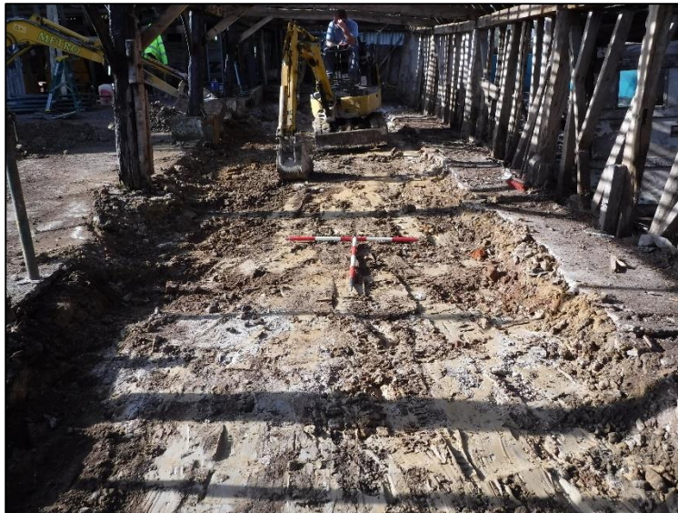
Plate 7: Natural directly below floor in cart shed
