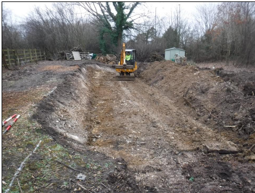
Plate 3: Working shot looking south-west showing dwelling footprint and line of old A24.
