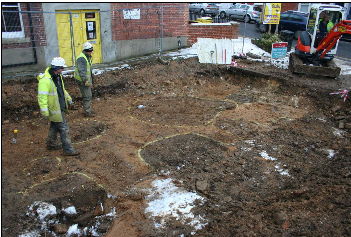
Plate 2: 5 East Street, Lewes: Features marked out on west side of site after topsoil strip
