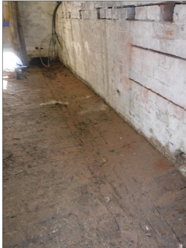
Plate 1: Gully running alongside the northeast wall
