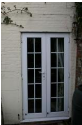
Plate 1 Tower House Scar in brickwork.
