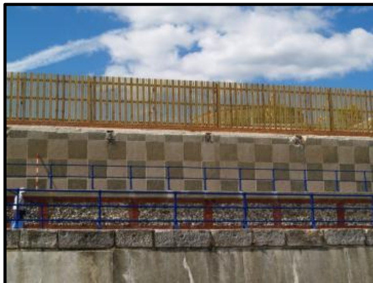
Plate 4: The Cantilever Balcony has been removed exposing the southern edge of the concrete slab and ends of its supporting RSJ's.
