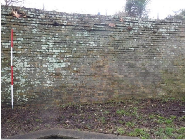
Plate 9: The counter scarp wall looking west, showing the damage caused by plants
