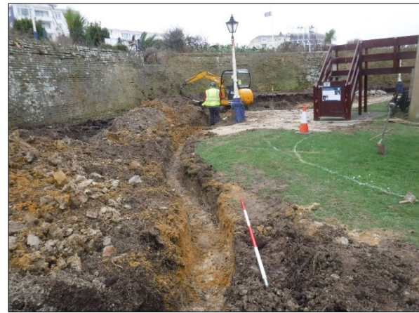
Plate 4: The Site looking northwest showing the footing trench for the new retaining wall
