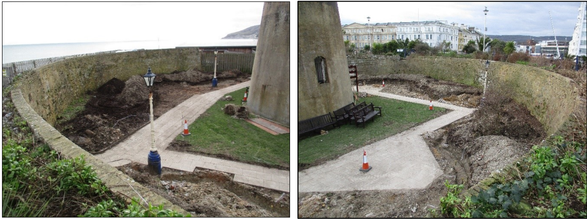
Plates 1 & 2: General views of the Site looking south and southwest, showing the groundworks
