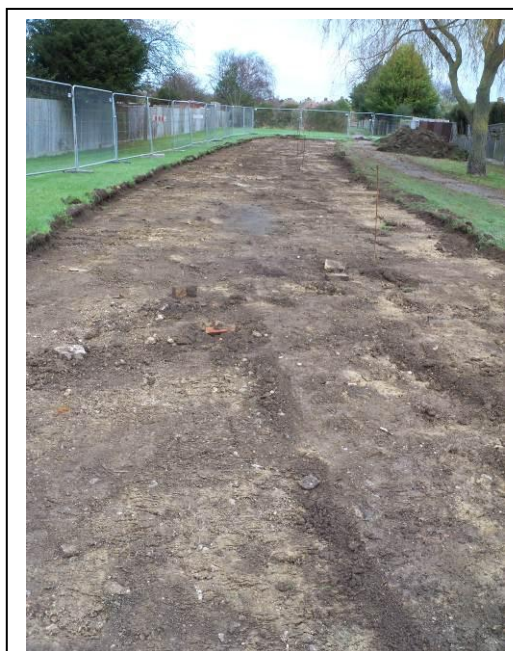
Plate 1: Ringwood Road to Bridge 3 Section looking NE, note how no impressions of the original track remain.
