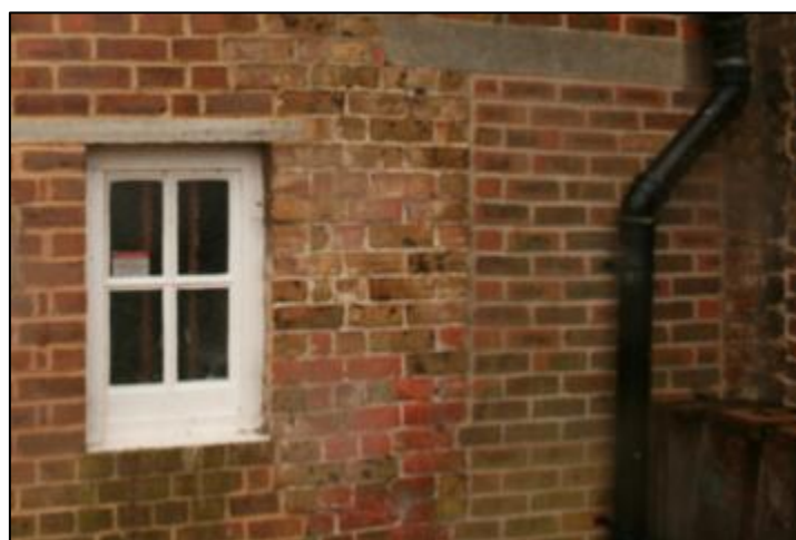
Plate 1: 224 High Street: Scar of earlier entrance in north wall of the north- eastern extension.
